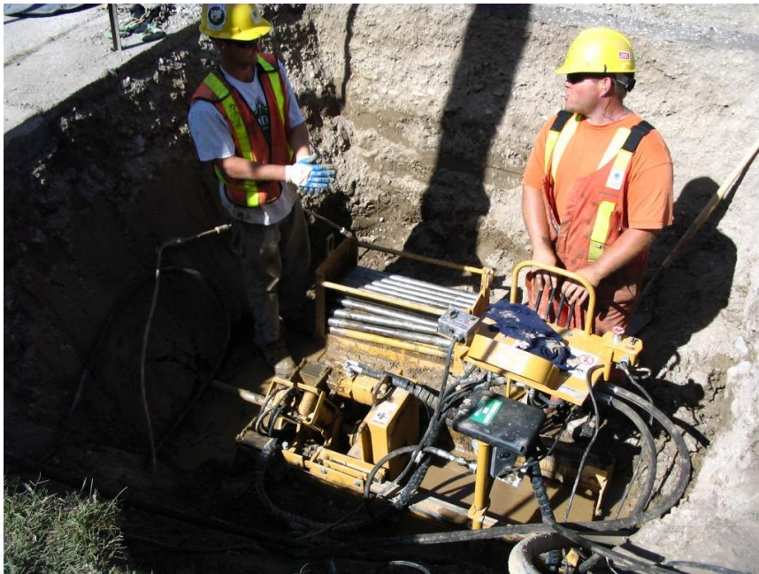
Trenchless installation of a new replacement main utilizing a directional drill unit
