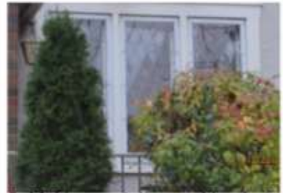
6. Multi-paned diamond leaded front windows and decorative quarry (main front window shown)
