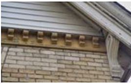
8. The gable is supported by wooden end brackets and a modillion course beneath
