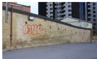
18. The washhouse, brick on a rubble stone foundation, slopes down towards the former creek-bed of Carling's Creek.
