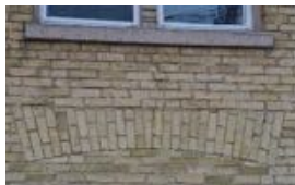
11. On the second storey of the front façade are double windows, which were apparently echoed on the first storey
