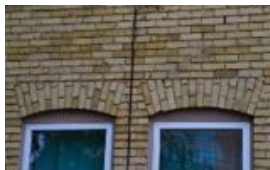
10. The fenestration is symmetrical within the irregular profile; with most of the principal windows being segmental-arched topped with brick voussoirs
