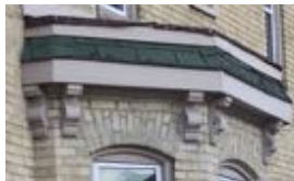
13. The bay is topped by a flat roof and the fascia board is decoratively supported by small brackets or modillions
