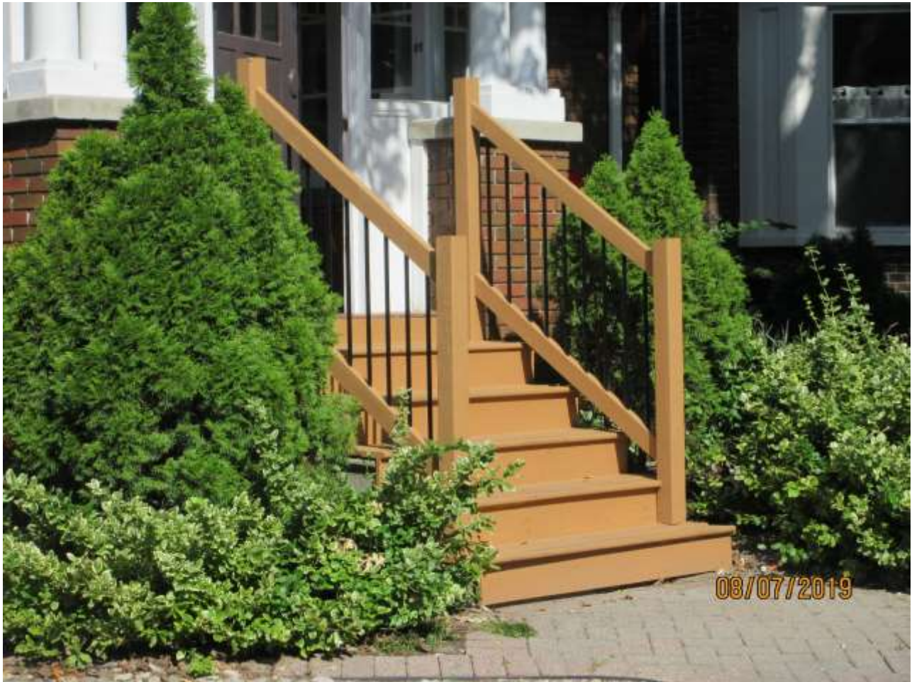
Image 3: Detail photograph of the new front steps of the property at 59 Wortley Road.
