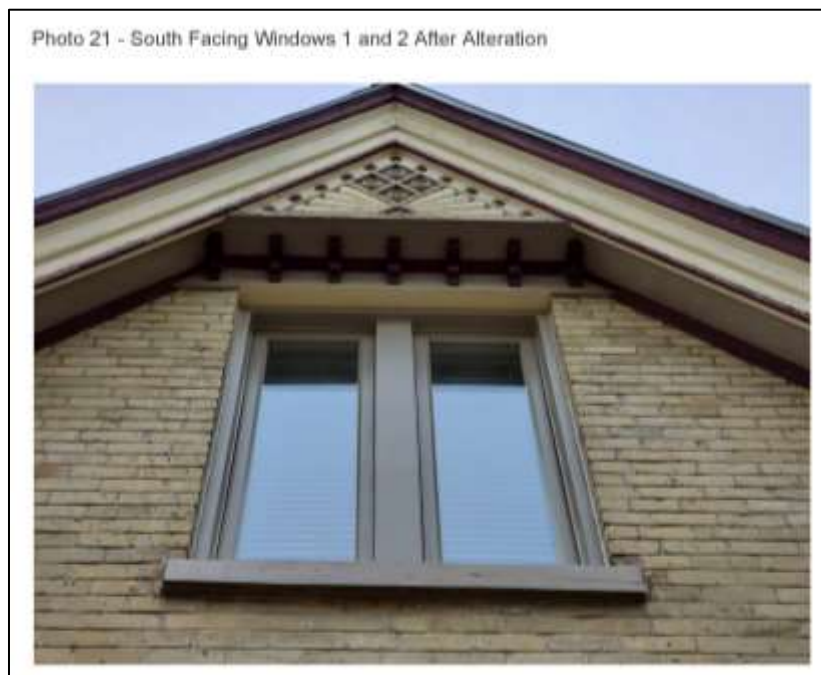
Image 13: Image of the south facing window 1 and 2 after the alteration (exterior), submitted as part of the Heritage Alteration Permit application. The mullion between the windows appears to have been removed or clad in siding.
