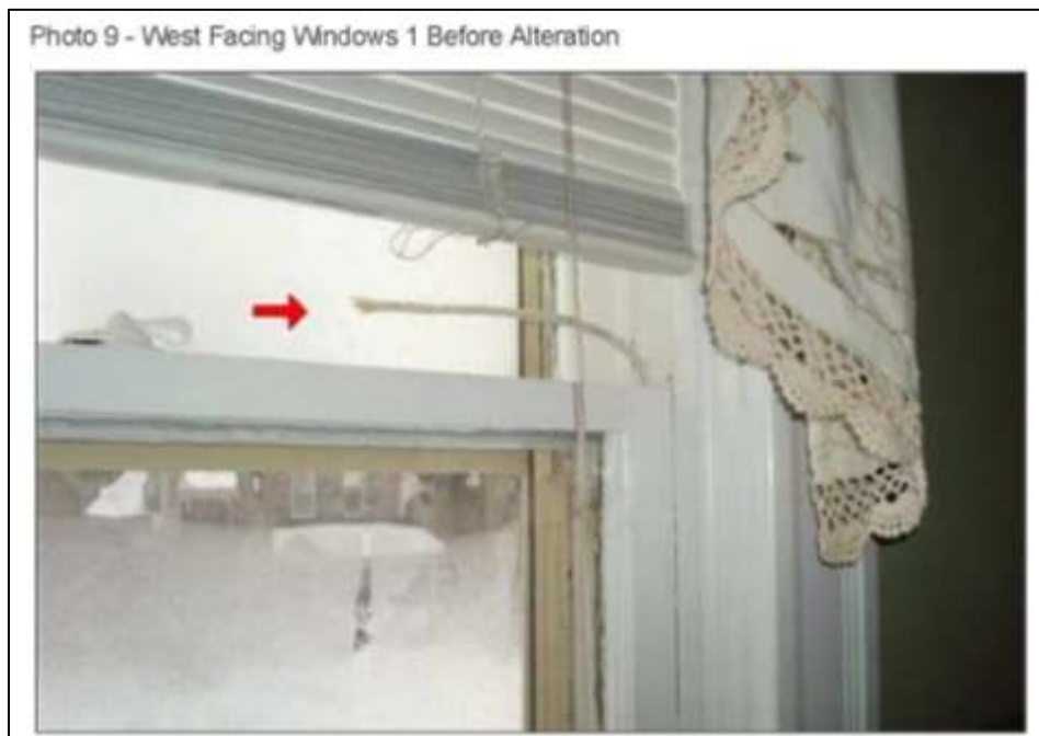
Image 6: Image, submitted as part of the Heritage Alteration Permit application, showing a cut or broken sash cord.
