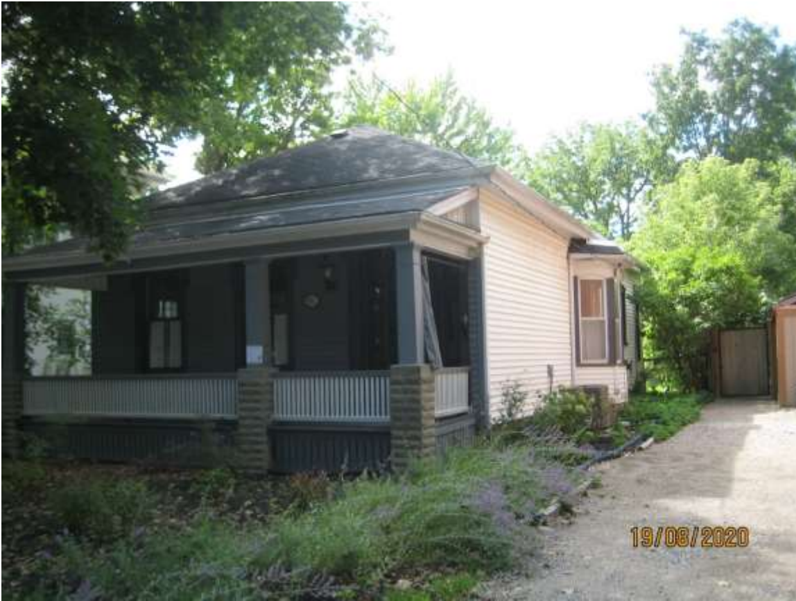
Image 5: Photograph showing the front (north) and side (west) facades of the dwelling, showing its existing conditions and various vinyl siding.
