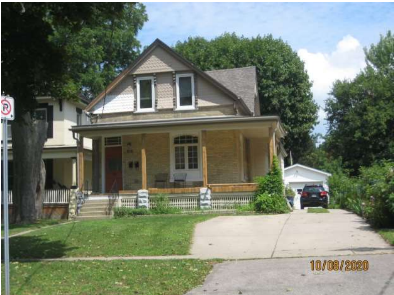
Image 4: Photograph showing unapproved alterations underway at 562 Maitland Street in August 2020. Note, the porch floor has been installed, and six 6" x 6" structural posts have been installed to support the porch roof.
