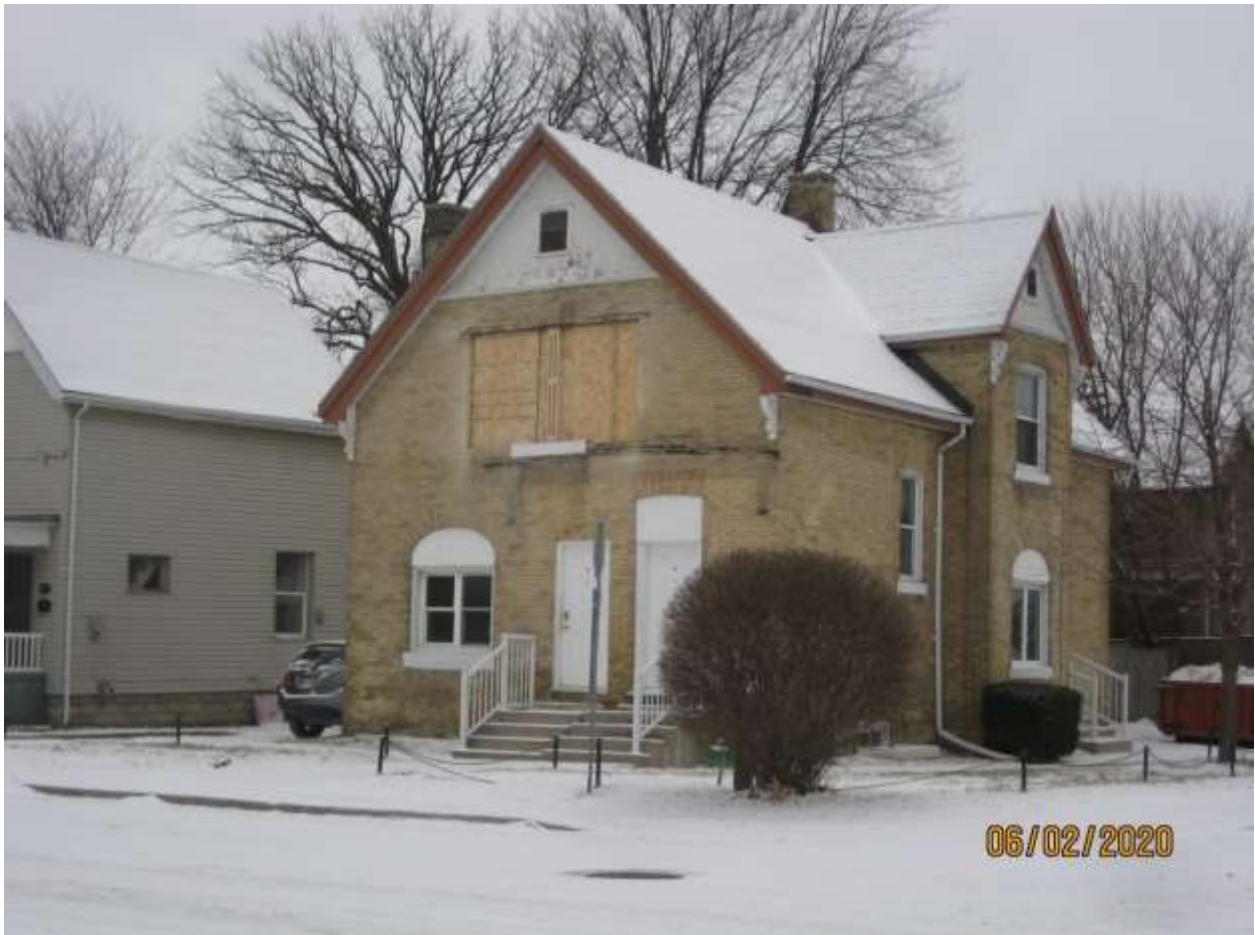
Image 3: Photograph showing unapproved alterations underway at 512 English Street in February, 2020. The plywood hoarding was installed in February, 2020, and has remained in this state, awaiting HAP approval.
