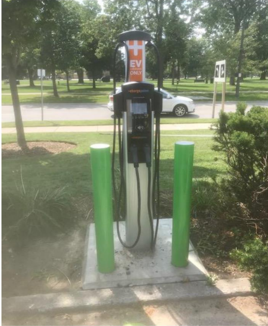
Sample of a Level 2, Dual EV Charger mounted on a precast concrete base. (located at London life)
