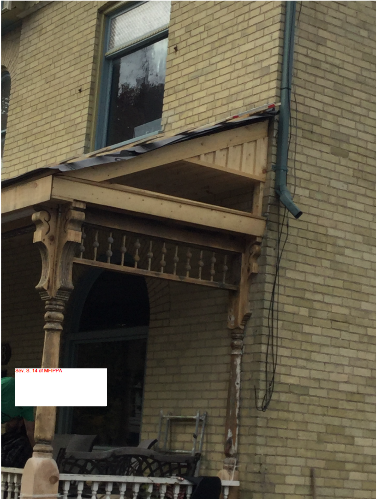
Image 7: Photograph submitted as a part of the Heritage Alteration Permit application for 938 Lorne Avenue showing detail of the porch design and existing spandrel details
