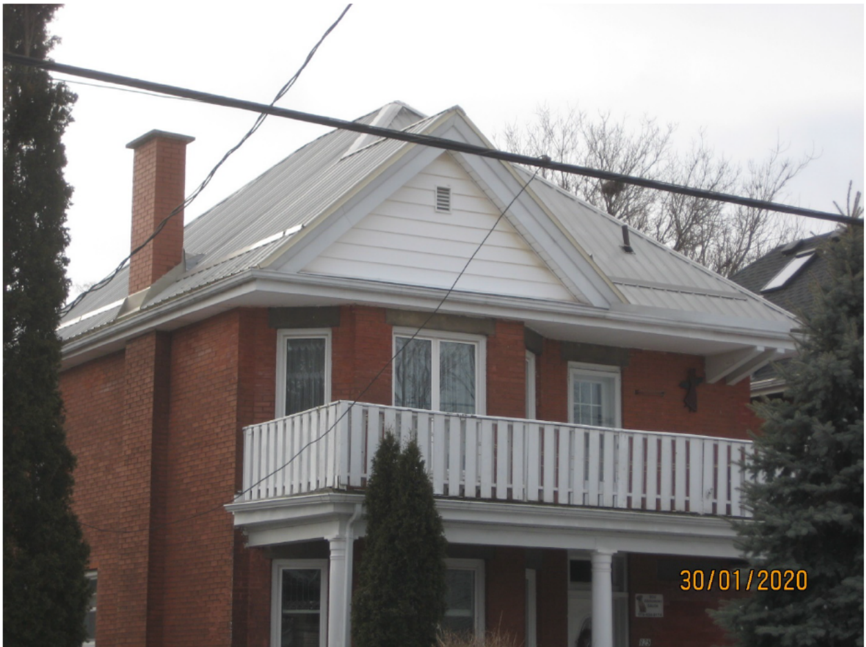
Image 14: Photograph showing unapproved sheet metal roofing material alteration at 825 Lorne Avenue in January 2020
