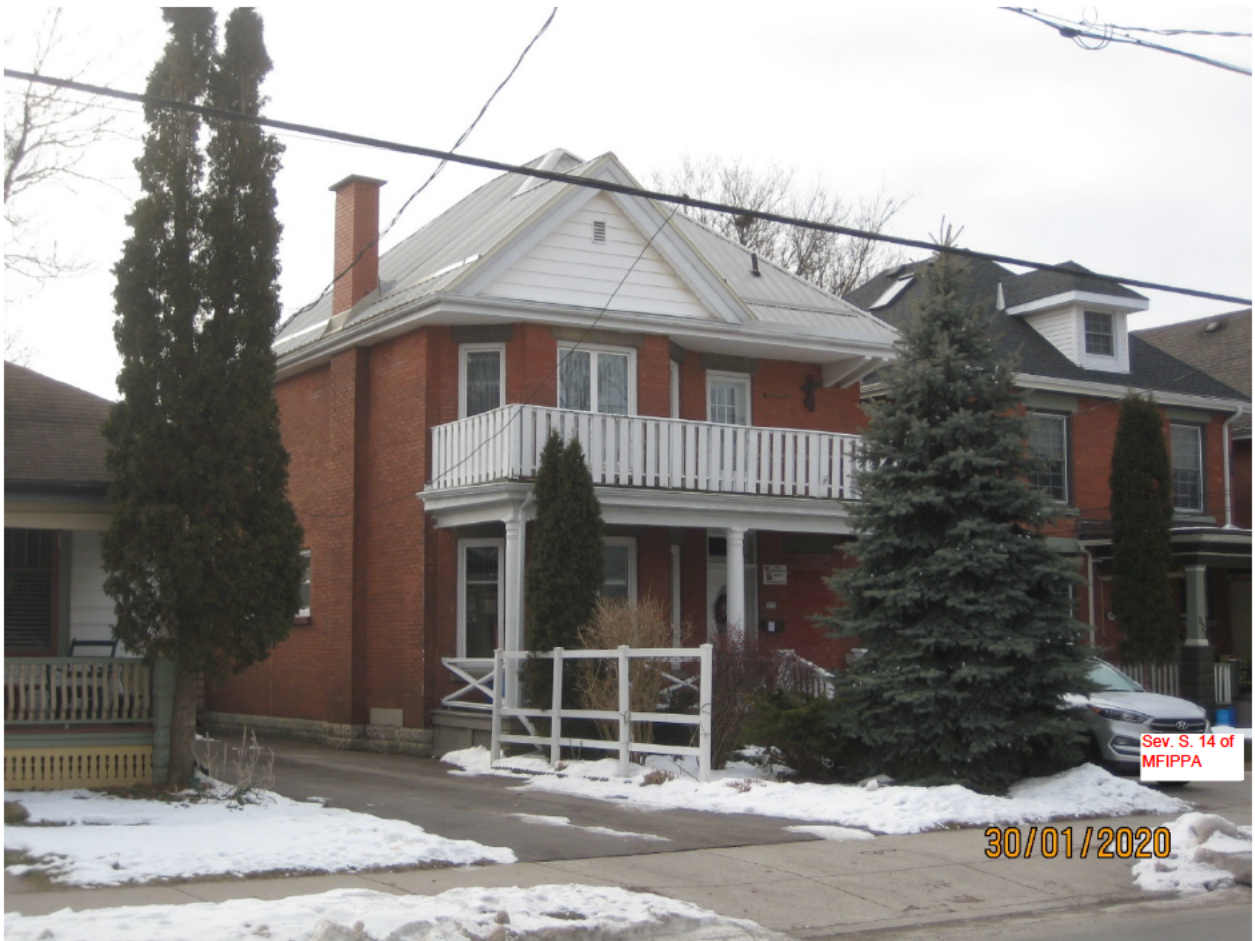
Image 13: Photograph showing unapproved sheet metal roofing material alteration at 825 Lorne Avenue in January 2020
