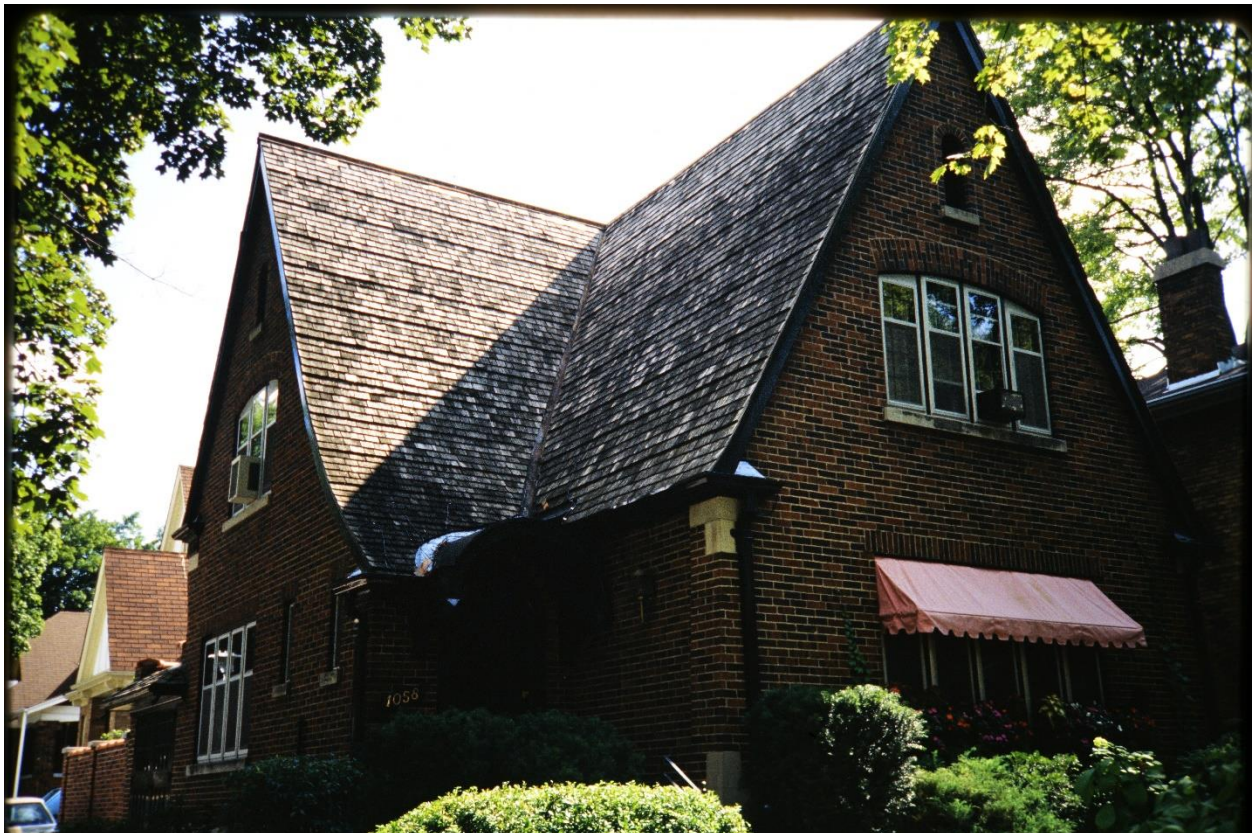
Image 2: Detail photograph of the property at 1058 Richmond Street, emphasizing the wood shingle roof (c.1990).
