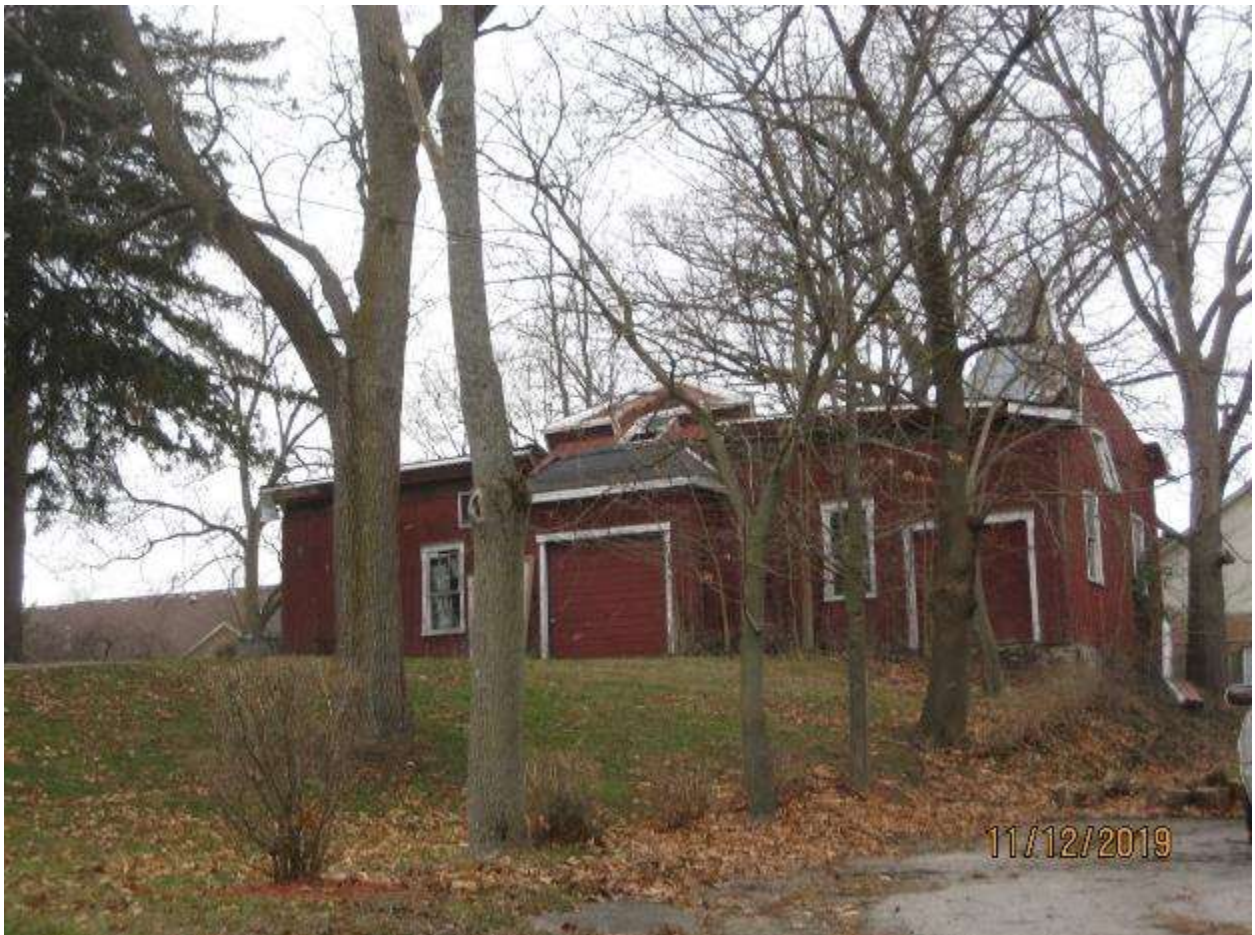
Image 32: Photograph showing the east side of the accessory building as viewed from Halls Mill Road, showing the collapse of the roof framing, December 11, 2019.
