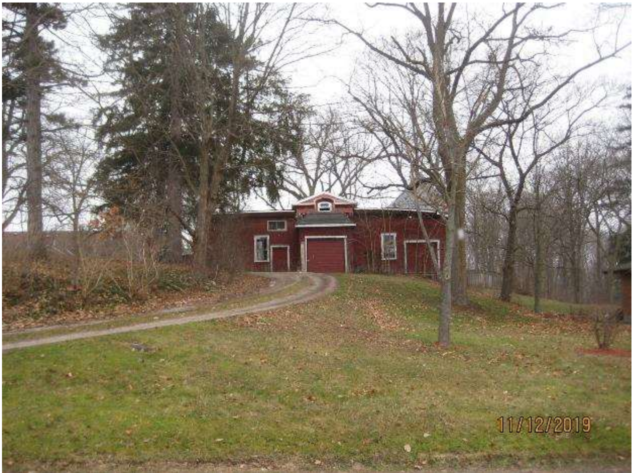
Image 30: Photograph showing the east side of the accessory building as viewed from Halls Mill Road, showing the collapse of the roof framing, December 11, 2019.
