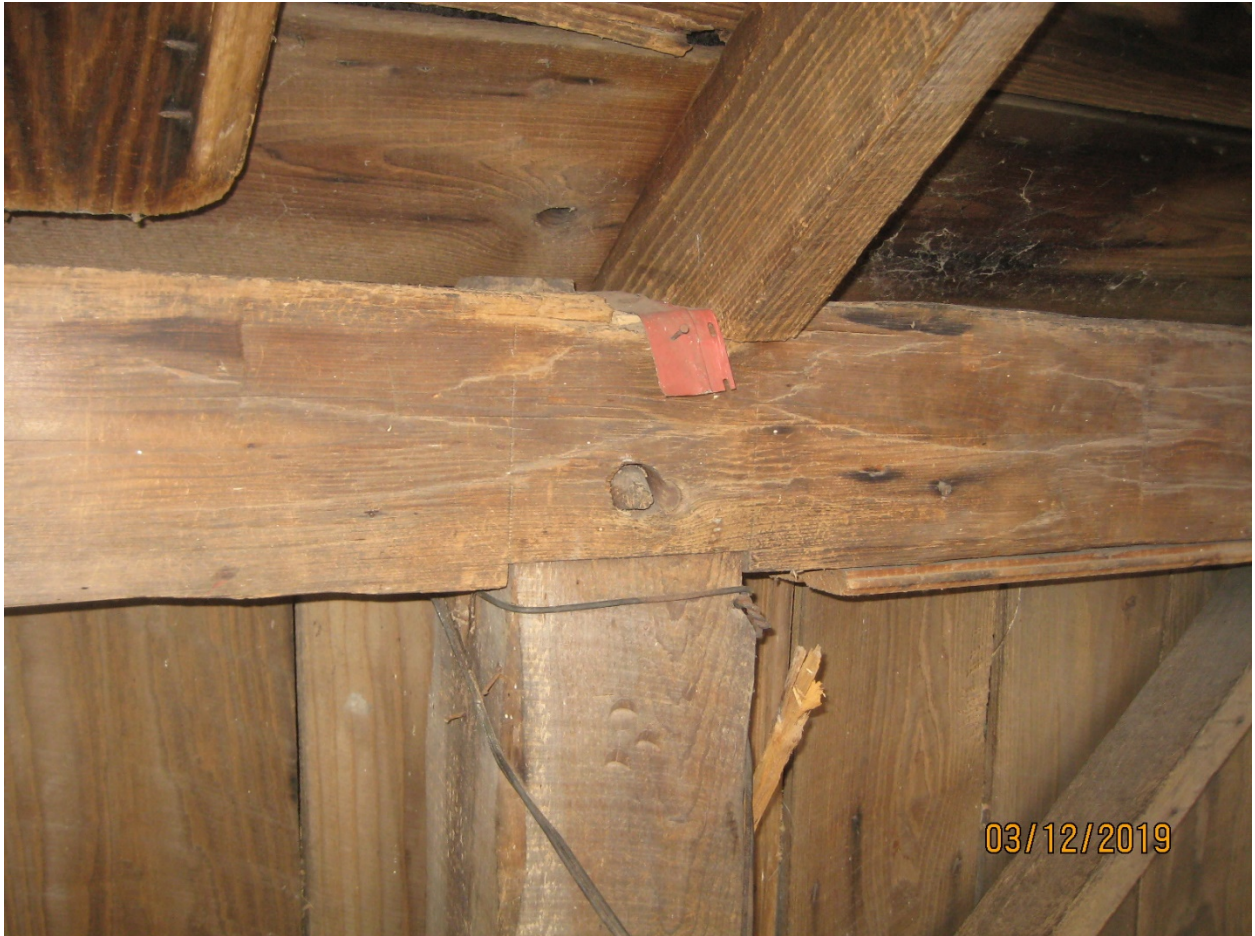
Image 29: Interior detail showing traditional mortise and tenon timber frame connections used throughout the accessory building, December 3, 2019.
