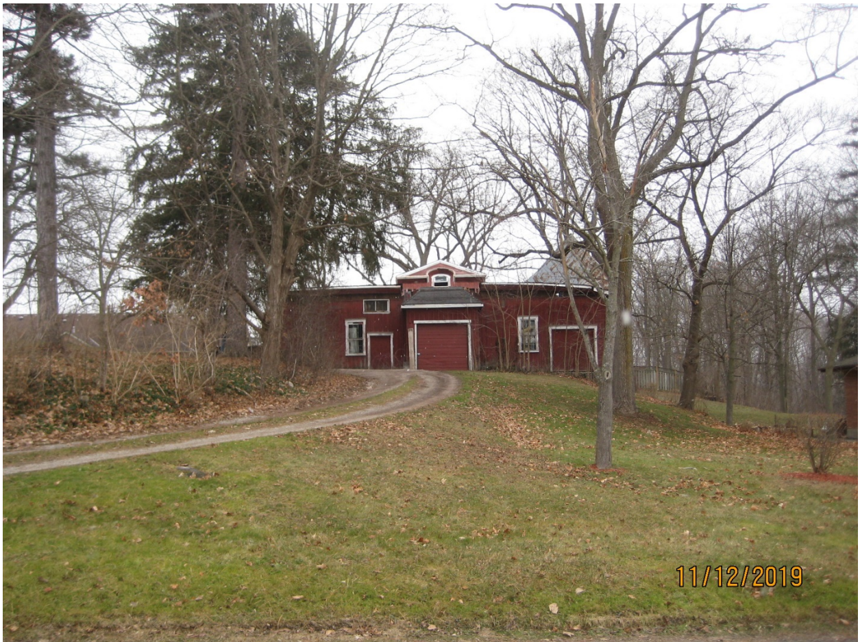
Image 30: Photograph showing the east side of the accessory building as viewed from Halls Mill Road, showing the collapse of the roof framing, December 11, 2019.
