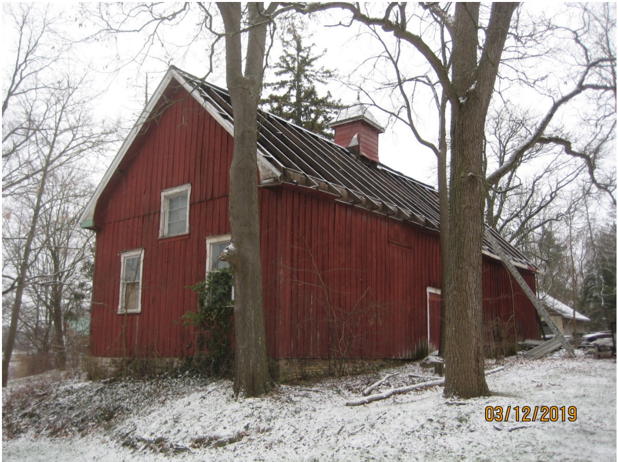
Image 23: Photograph of the west side of the accessory building, showing the removed roof sheathing, December 3, 2019.
