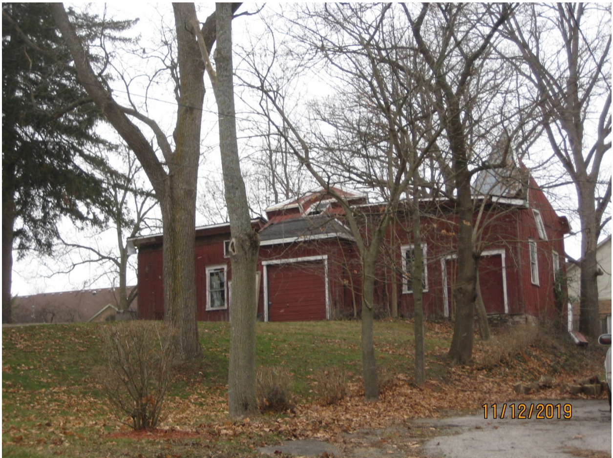
Image 32: Photograph showing the east side of the accessory building as viewed from Halls Mill Road, showing the collapse of the roof framing, December 11, 2019.
