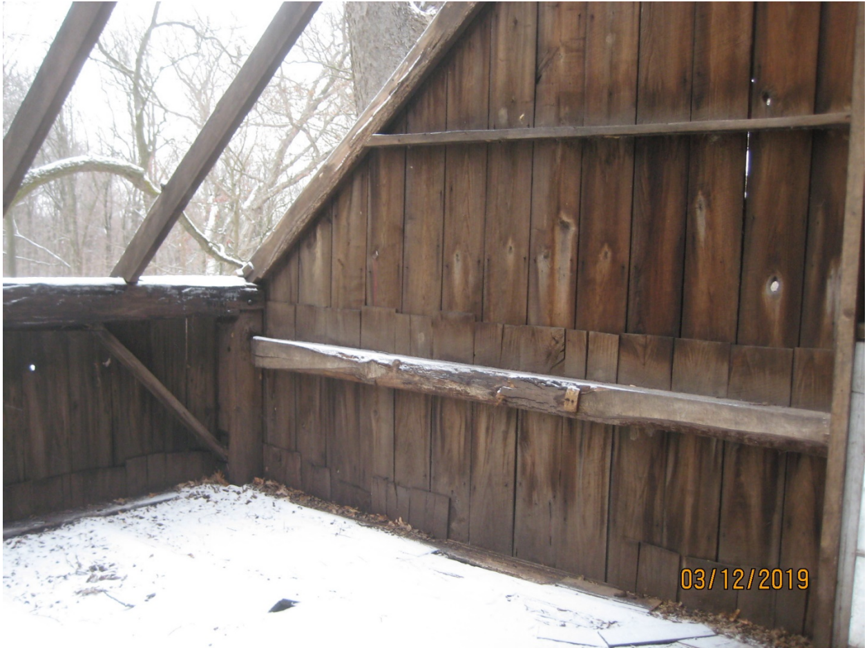
Image 27: Interior detail of the mortise and tenon timber frame construction of the accessory building, December 3, 2019.
