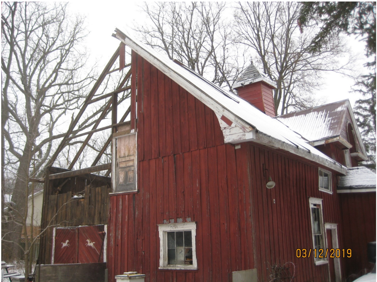
Image 22: Photograph of the south side of the accessory building. Note the portions of the exterior cladding and roof had been removed by the property owner the in the fall of 2019, December 3, 2019.
