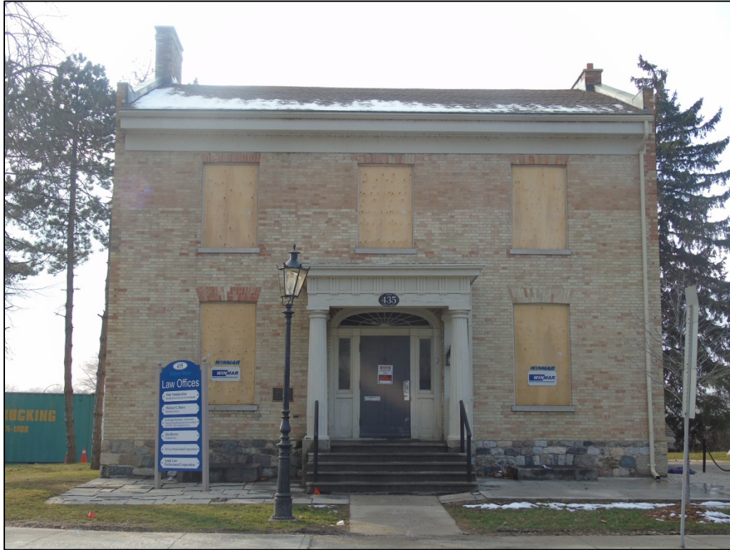
Image 1: View showing heritage structure at 435 Ridout Street North, with boarded-up windows due to fire damage from September 2018
