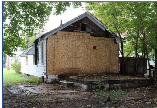
5. (bottom left) South elevation with collapsed rear roof.
