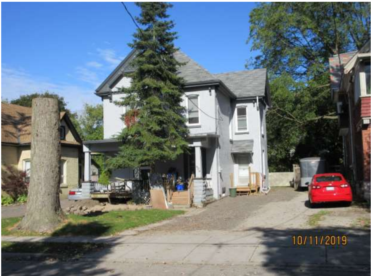
Image 2: Photograph of the property at 906 Lorne Avenue showing unapproved alterations underway, photographed on October 11, 2019.
