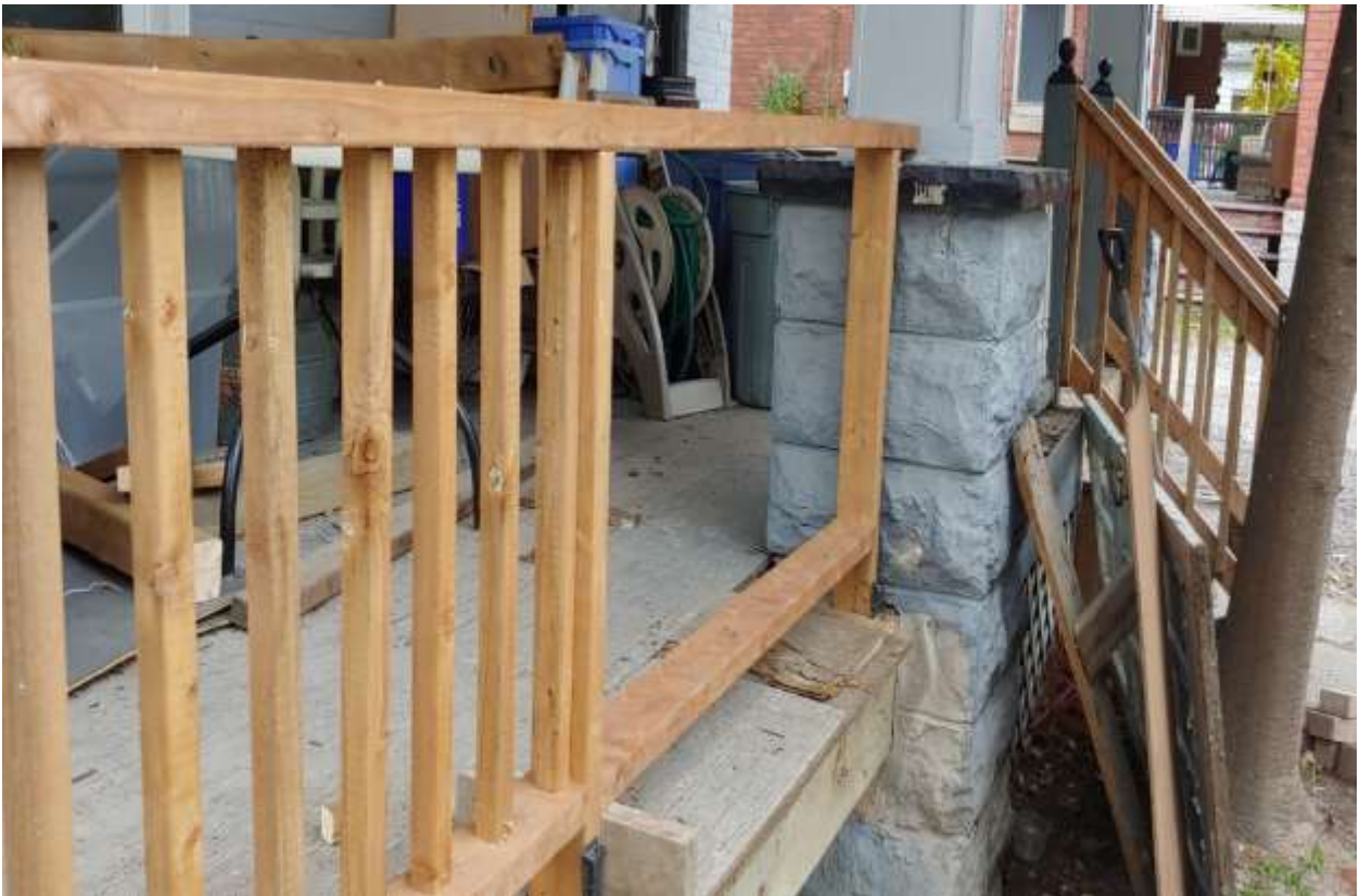
Image 6: Photograph showing proposed railing and square spindle alterations to the porch at 906 Lorne Avenue, submitted as a part of the Heritage Alteration Permit application (October 2019). Note, the new height of the top rail will be required in order to meet the requirements of the Ontario Building Code.
