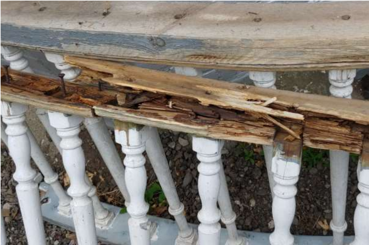
Image 3: Detail of the top and bottom rails on the porch at 906 Lorne Avenue submitted as a part of the Heritage Alteration Permit application, showing the deteriorated wooden elements (October 2019).
