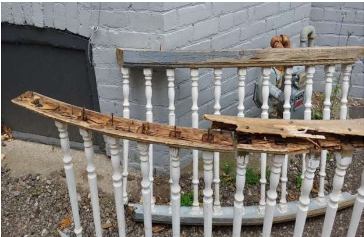
Image 4: Photograph of the top and bottom rails on the porch at 906 Lorne Avenue submitted as a part of the Heritage Alteration Permit, showing the deteriorated wooden elements (October 2019). Note, the railings are sitting upside down so the rotted bottom rail is most visible in the photograph.
