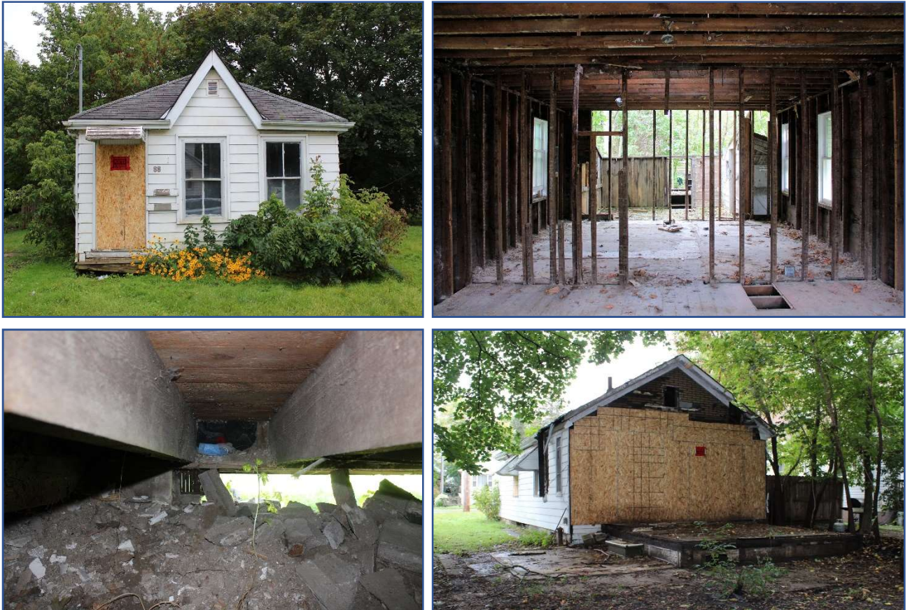
Clockwise from top Left 24. North elevation of 88 Blackfriars Street. 25. Interior view of the gutted interior of 88 Blackfriars, with the partially demolished rear exterior walls and roof. 26. View of the south elevation with temporary plywood sheathing as per City of London unsafe building order. 27. View of crawl space and mud sill floor framing and opening from collapsed foundation.
