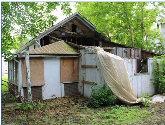
32. The above photograph shows the rear portions of the house in June 2019. These were removed as directed due to concern for public safety.
