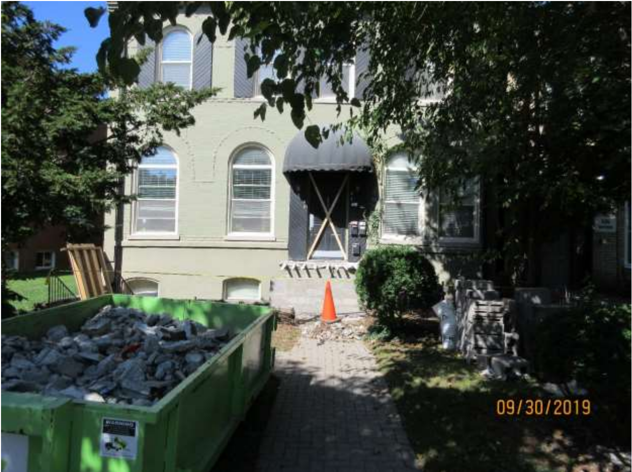
Image 5: Photograph of the property at 430 Dufferin Avenue on September 30, 2019 showing work underway.
