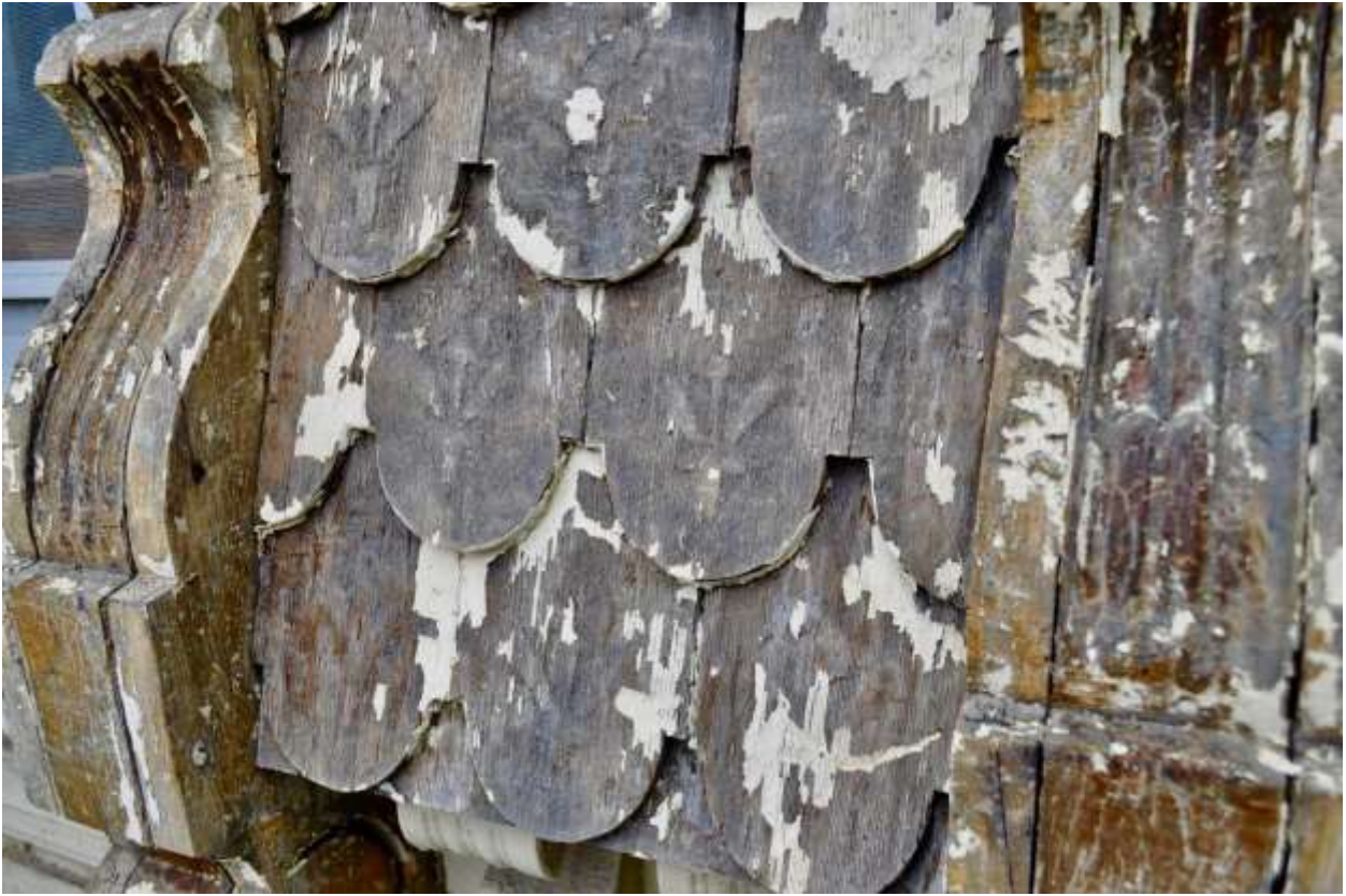
Image 4: Detail photograph of the wood shingle imbrication adjacent to the window openings in the second storey. Note the embossed foliage motif on the wood shingles, exposed during the restoration of the exterior woodwork. Photograph courtesy of A. Johnson.
