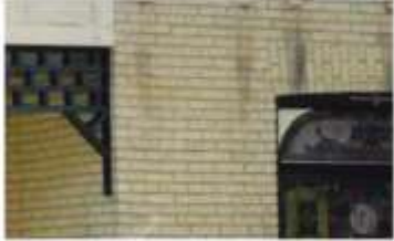
4. Buff brick veneer exterior cladding, with voussoirs above the window and door openings
