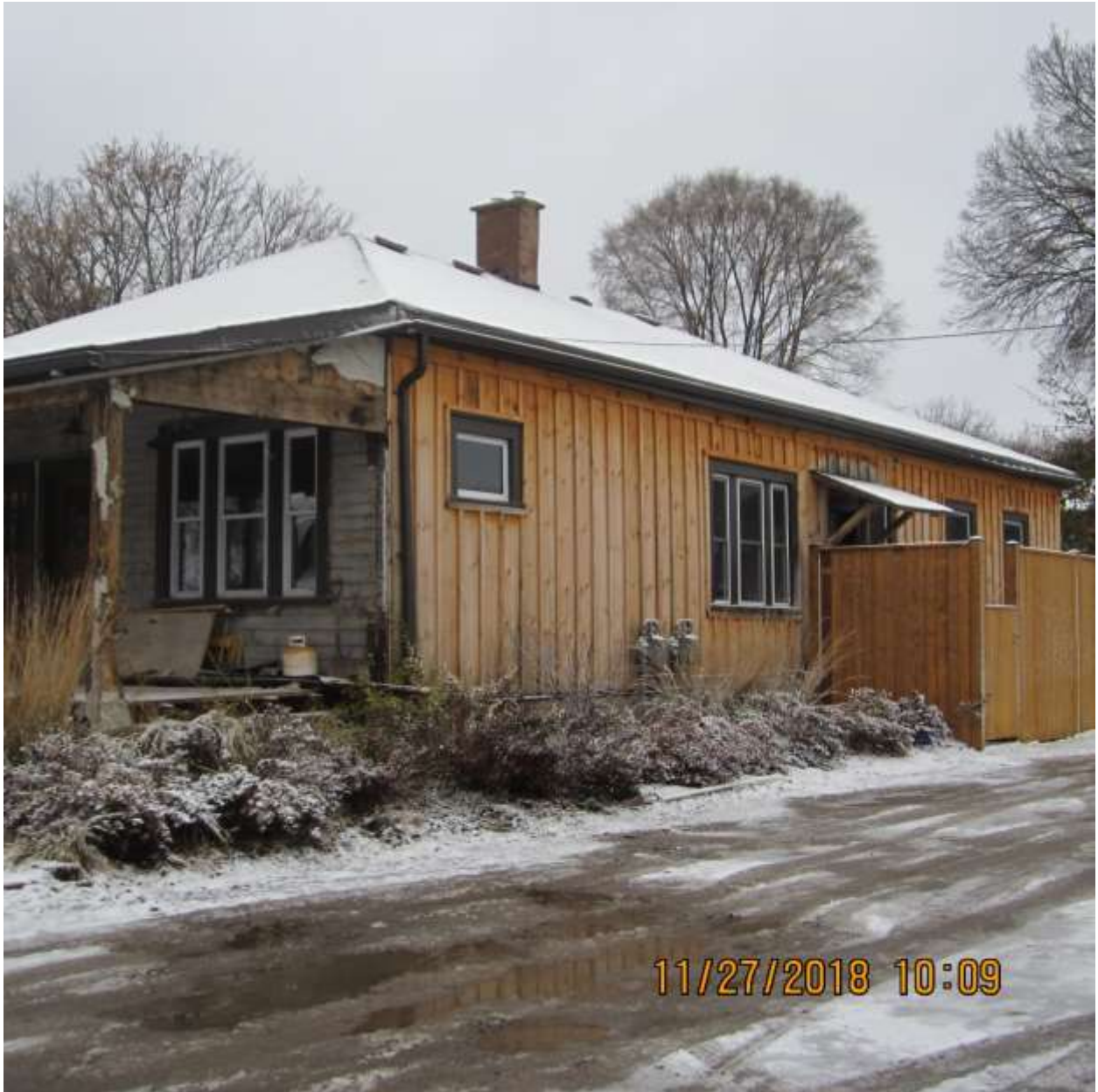
Image 3: Photograph of the property at 504-506 Maitland Street on November 27, 2018 showing unapproved alterations.
