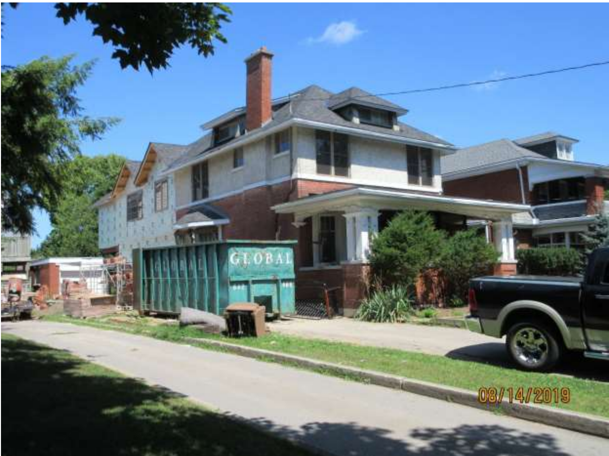
Image 4: Photograph showing the construction of the rear addition, and also the replacement of the windows on the second storey of the existing building on August 14, 2019. The rear addition was approved by HAP18-063-D, which excluded alterations to the existing building.
