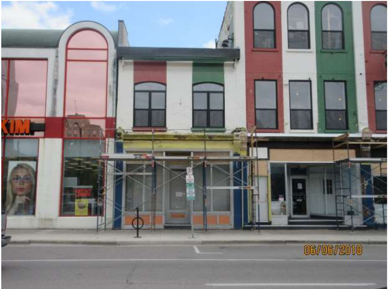
Image 3: Photograph showing alterations underway on June 6, 2018, including replacement of the windows on the upper floor of the building at 213 King Street.
