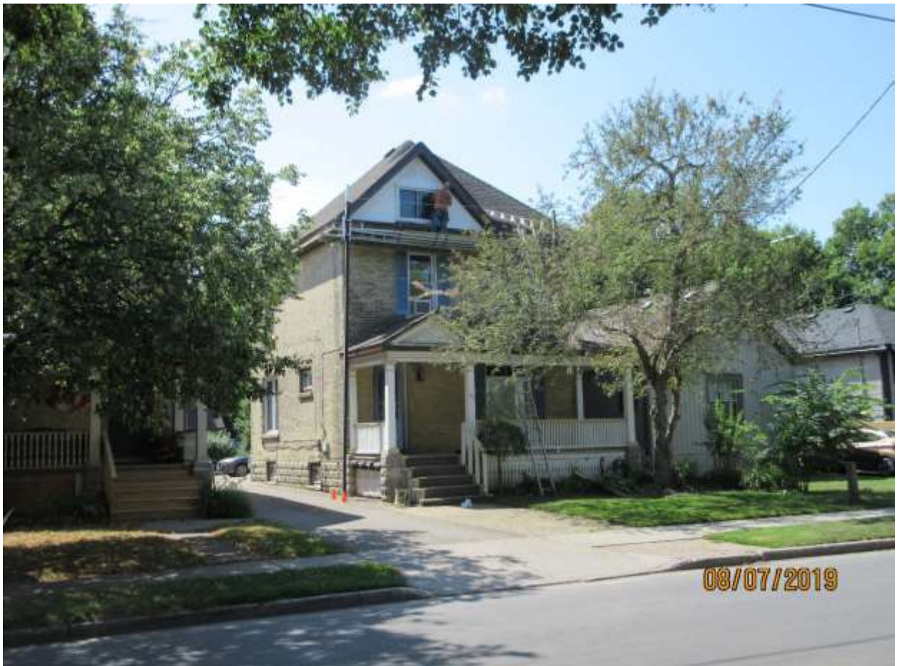
Image 4: Photograph showing unapproved alterations underway at 40 Craig Street on August 7, 2019.
