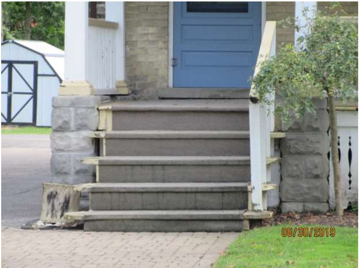
Image 6: Detail photograph of the existing conditions of the front steps of the building at 40 Craig Street.
