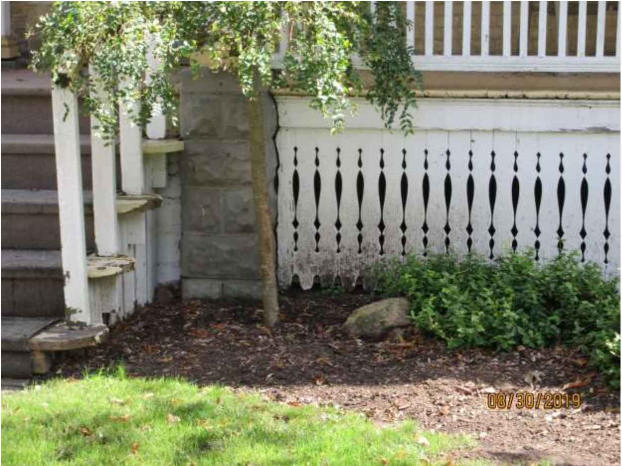
Image 7: Detail photograph of the existing conditions of the front steps and porch skirt of the building at 40 Craig Street.
