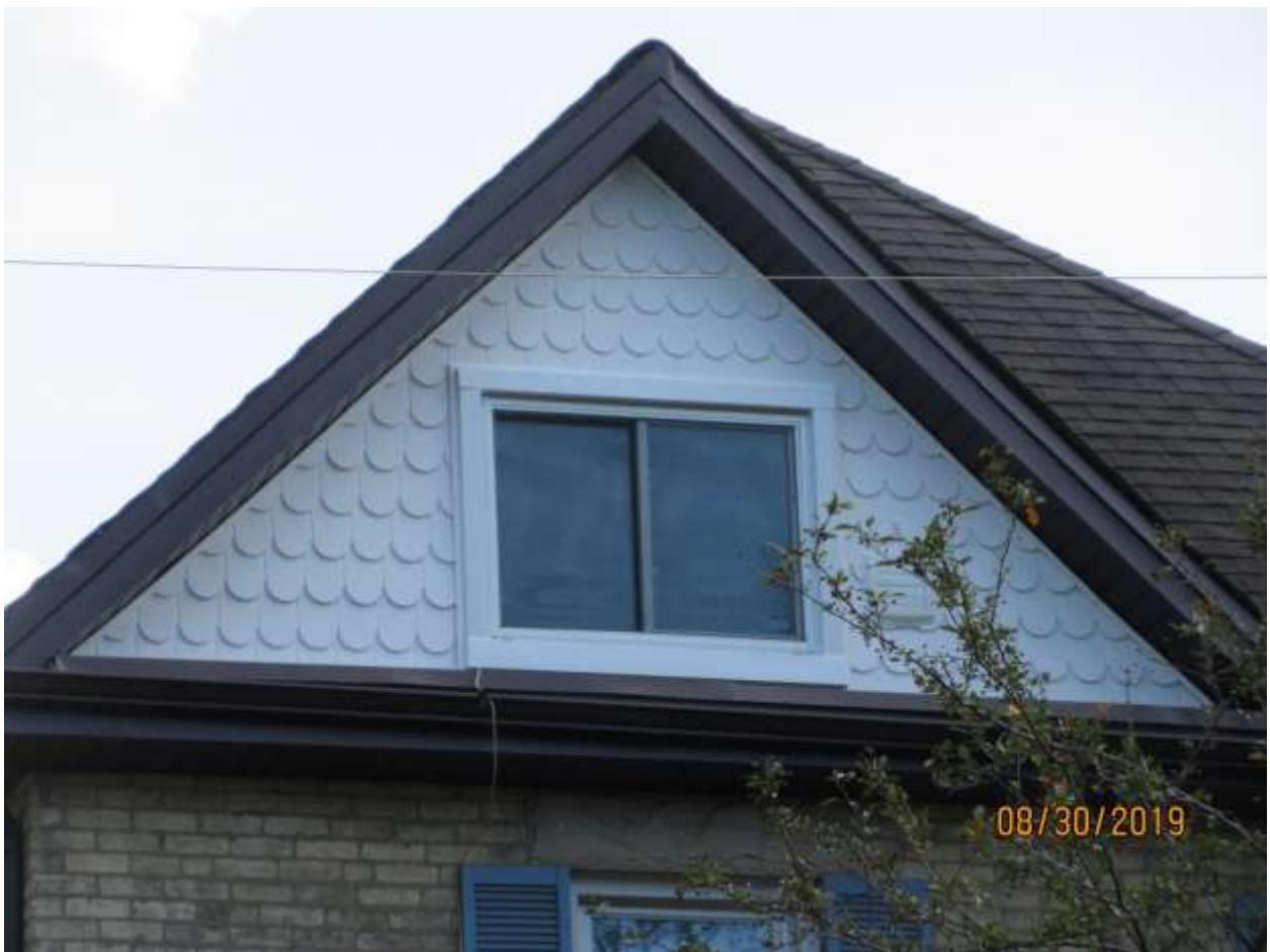
Image 5: Detail photograph of the gable of the building at 40 Craig Street with the vinyl scalloped shingles.
