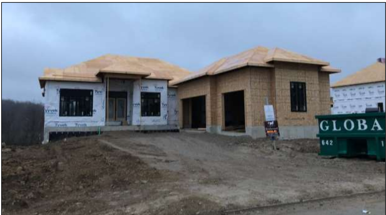
Figure 5: Example of 'L' shaped dwelling with active floor space in front of garage
