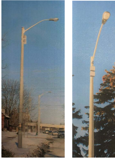
Figure 2: Photos of Ericsson small cells attached on concrete streetlight pole.
