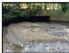
Photo 23: Sediment deposition downstream of Proudfoot Lane. The culvert is also full of sediment.
