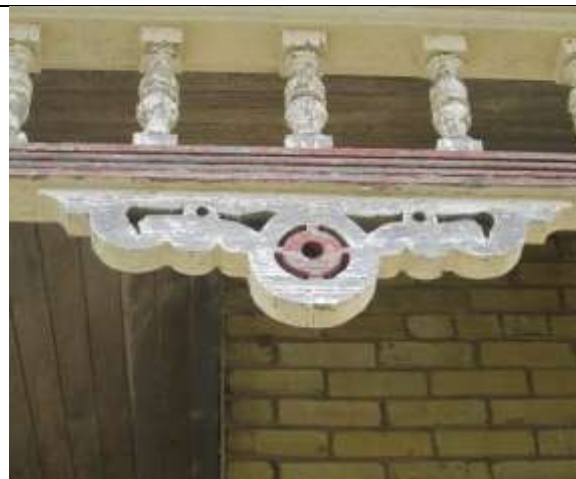
Image 23. Close up of verandah details. Front façade of the farmhouse located at 3303 Westdel Bourne. April 2019.
