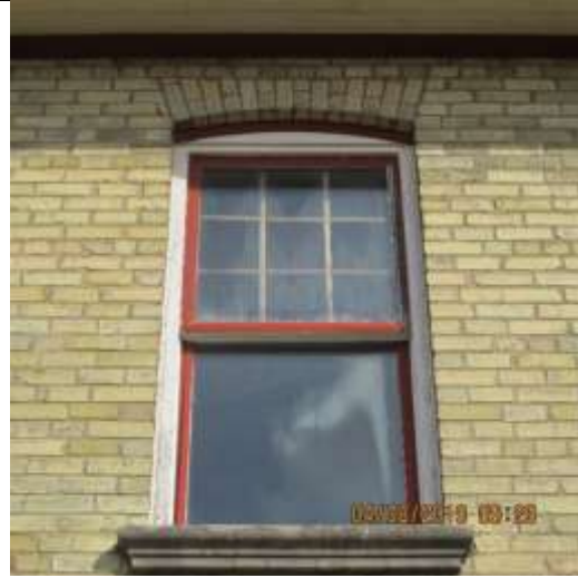
Image 13. Window example, south façade of the farmhouse located at 3303 Westdel Bourne, looking west. April 2019.
