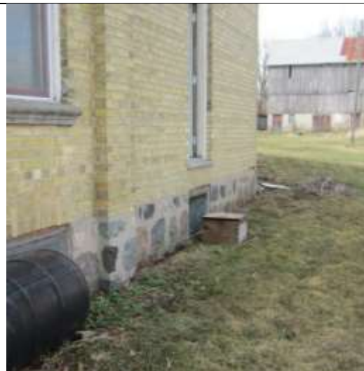
Image 15. Field Stone foundation, north façade of the farmhouse located at 3303 Westdel Bourne. April 2019.
