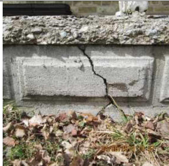
Image 25. Close of up of the concrete base of the verandah. Front façade of the farmhouse located at 3303 Westdel Bourne. April 2019.
