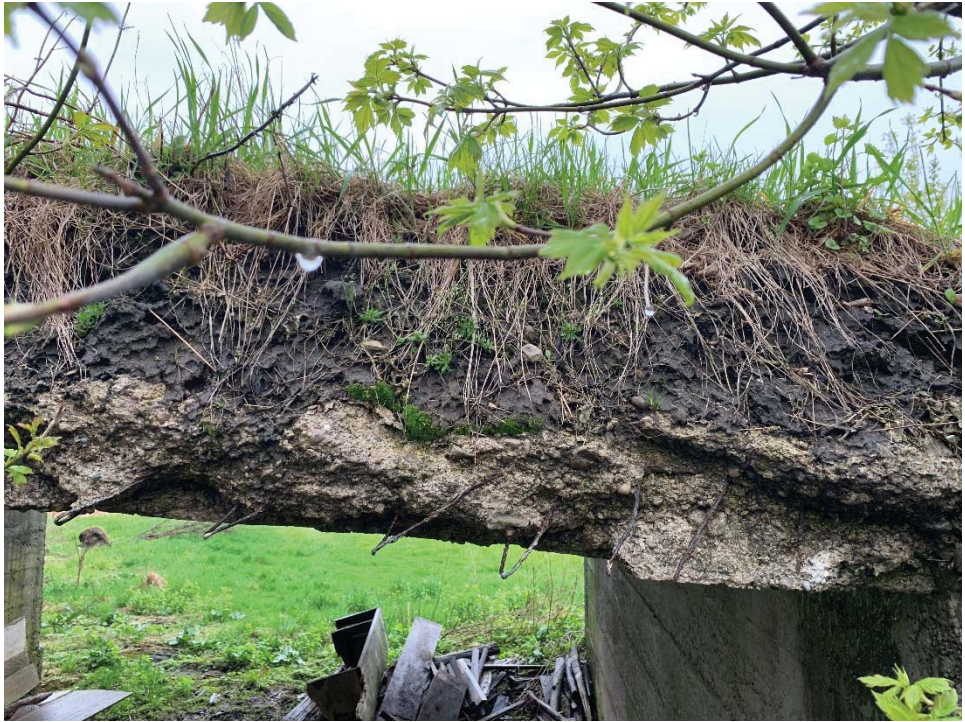
Figure 5.0 - Photo of Existing Ramp Structure with Severe Delamination/Corrosion
