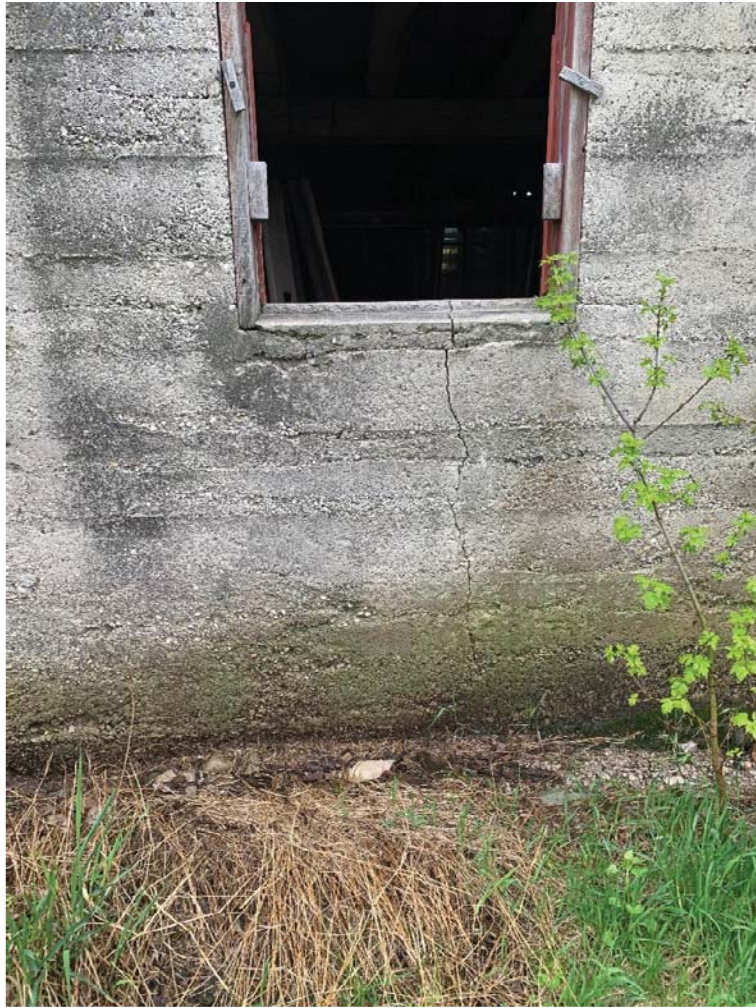
Figure 9.0 - Photo of Cracked Existing Foundation Wall
