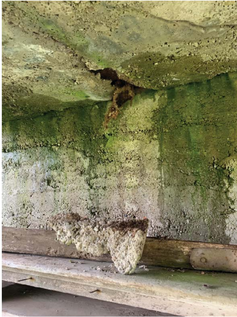
Figure 4.0 - Photo of Existing Ramp Structure with Severe Pitting/Spalling/Delamination
