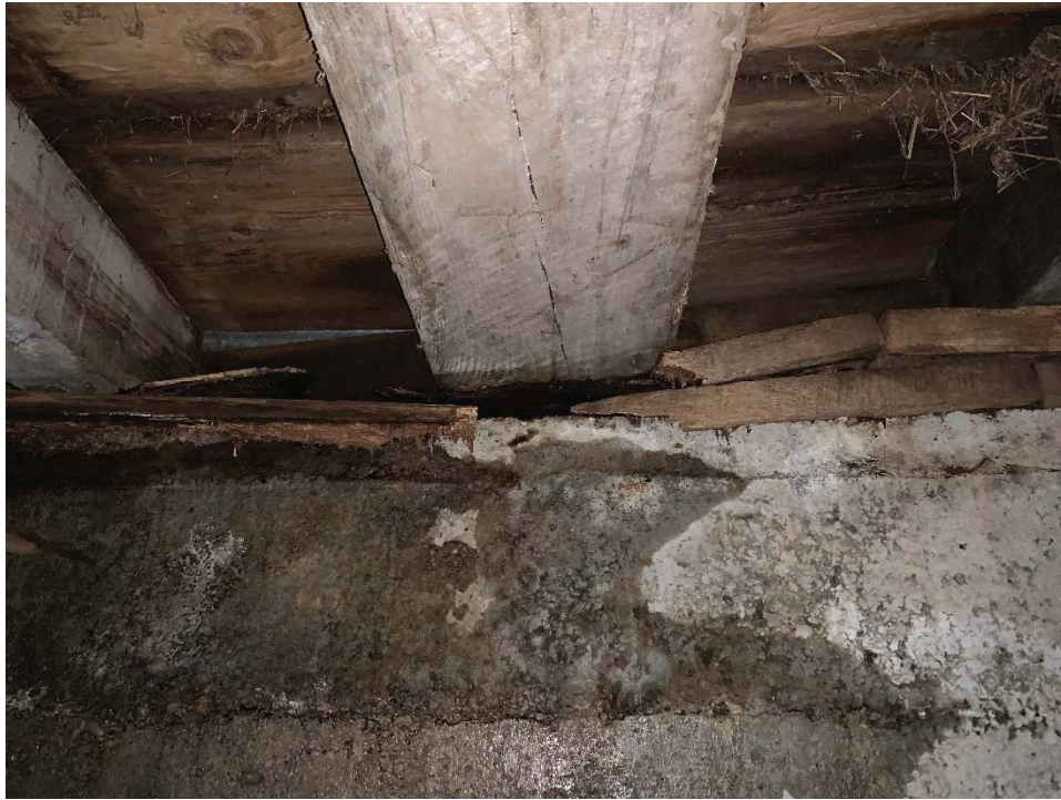
Figure 7.0 - Photo of Damaged Perimeter Sill-plate
