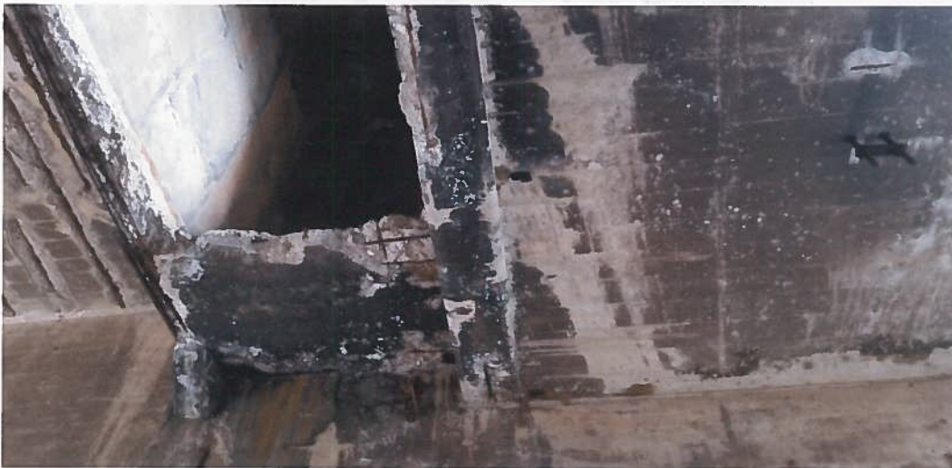
Photo No 05: Delaminated Concrete Beam at Link
