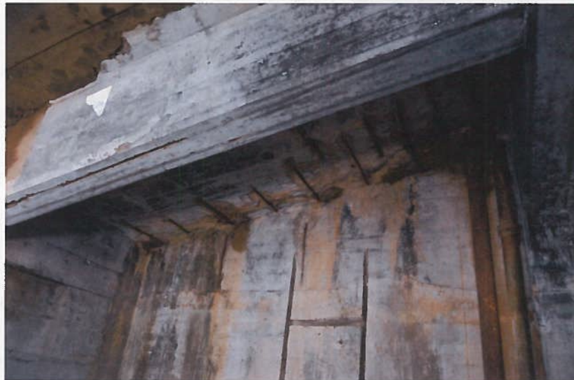
Photo No 11: Interior Suspended Slab (Delaminated Concrete)
