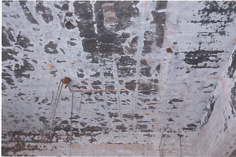
Photo No 10: Interior Suspended Slab (cracked along rebar)
