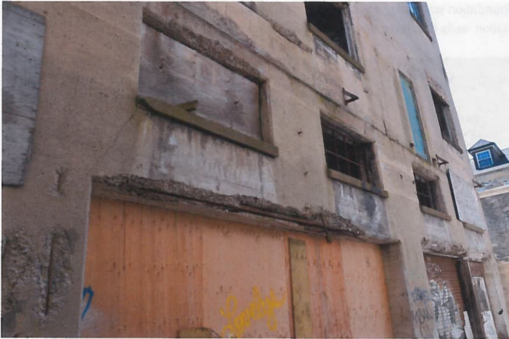
Photo No 04: Delaminated Concrete Beams
