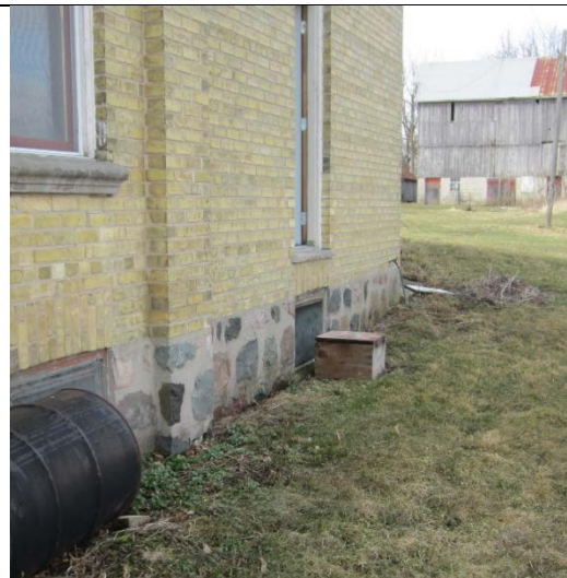
Image 15. Field Stone foundation, north façade of the farmhouse located at 3303 Westdel Bourne. April 2019.
