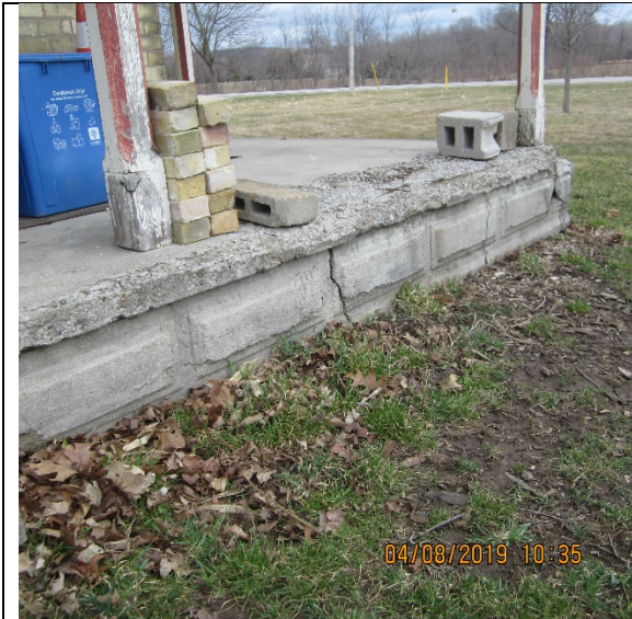
Image 24. Verandah concrete base. Front façade of the farmhouse located at 3303 Westdel Bourne. April 2019.
