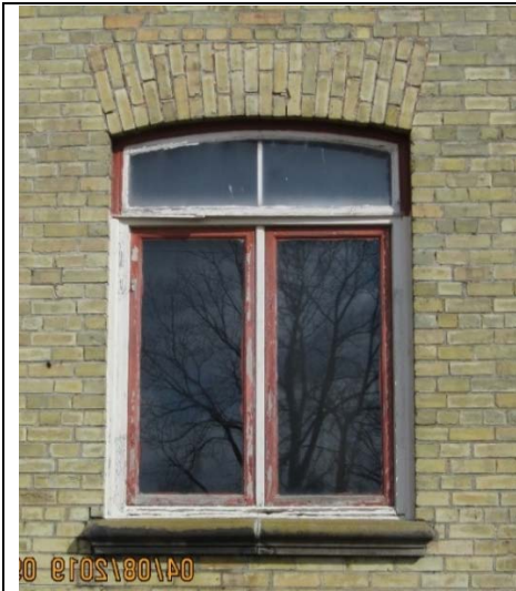
Image 12. Window example, front façade of the farmhouse located at 3303 Westdel Bourne. April 2019.
