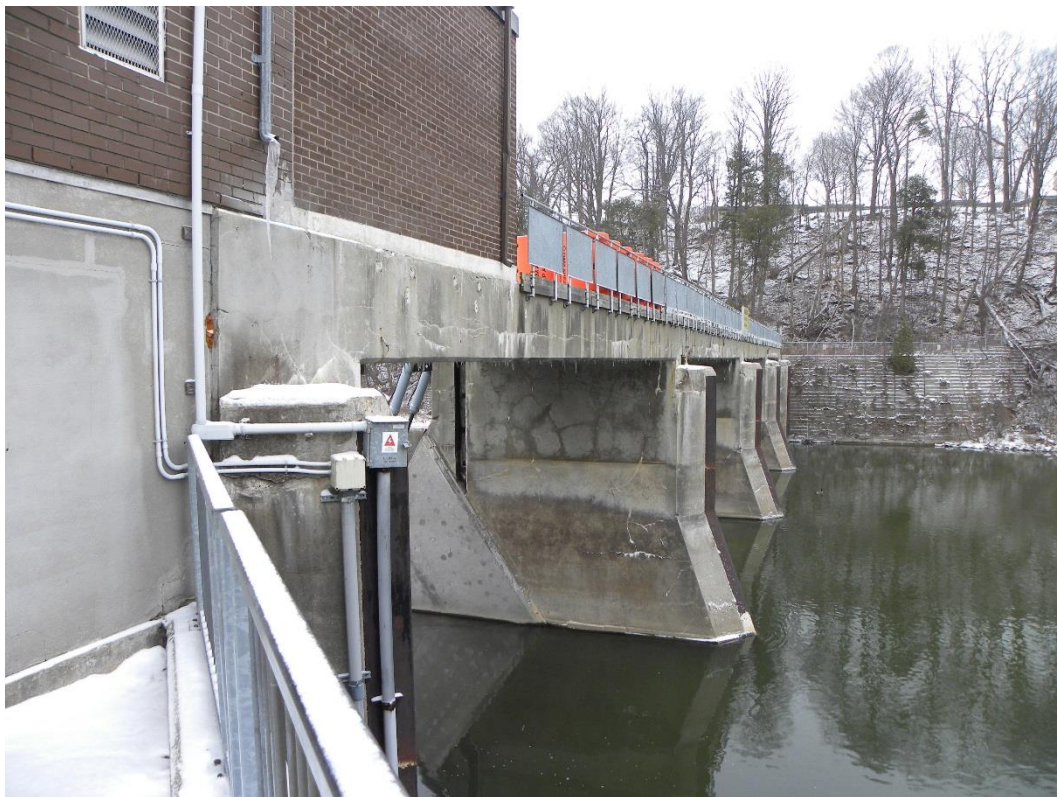
Figure 17: Vertical stop log groove (centre) on the southeast side of the spillway pier (January 18, 2019).
