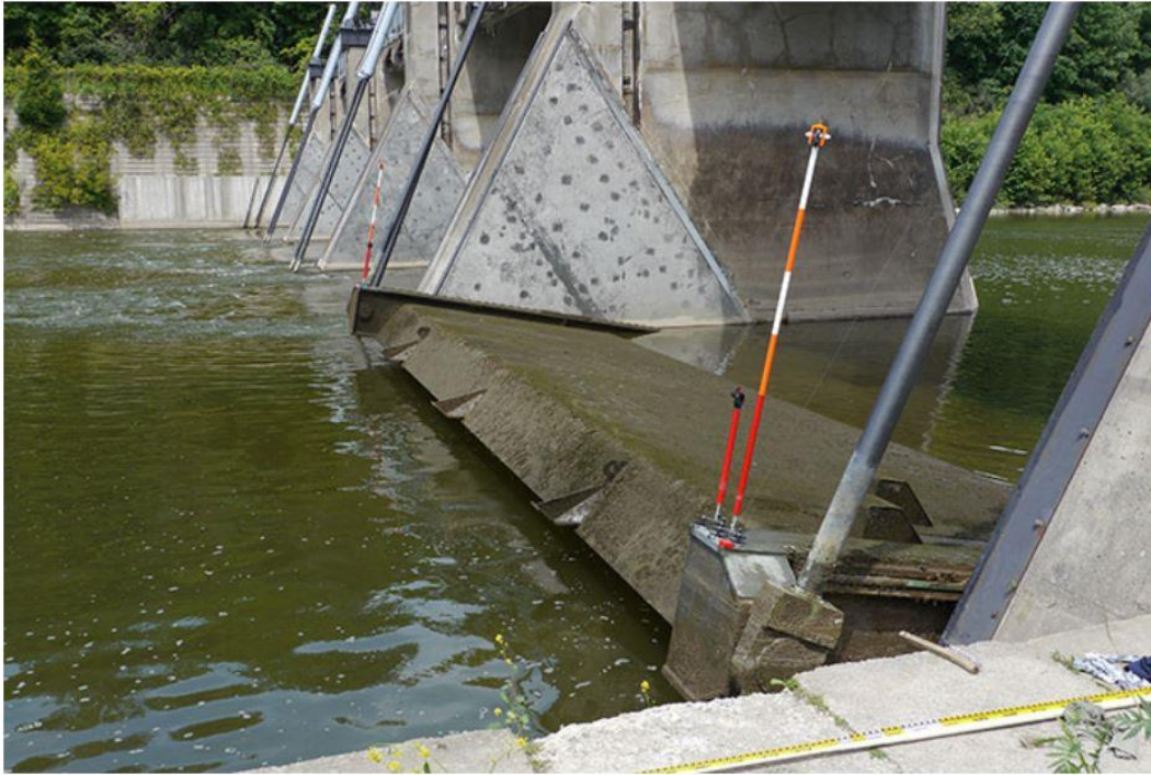
Figure 18: Tilting gates on the Springbank Dam (from City of London 2018).
