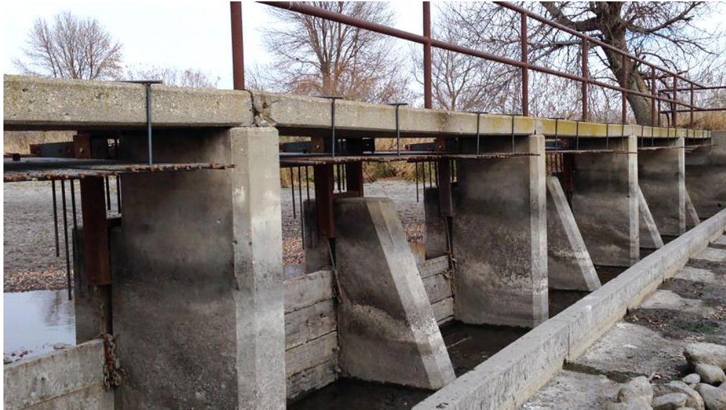
Figure 16: Example of stop log dam with buttresses in Lake Ocheda, Minnesota (Buntjer 2018).
