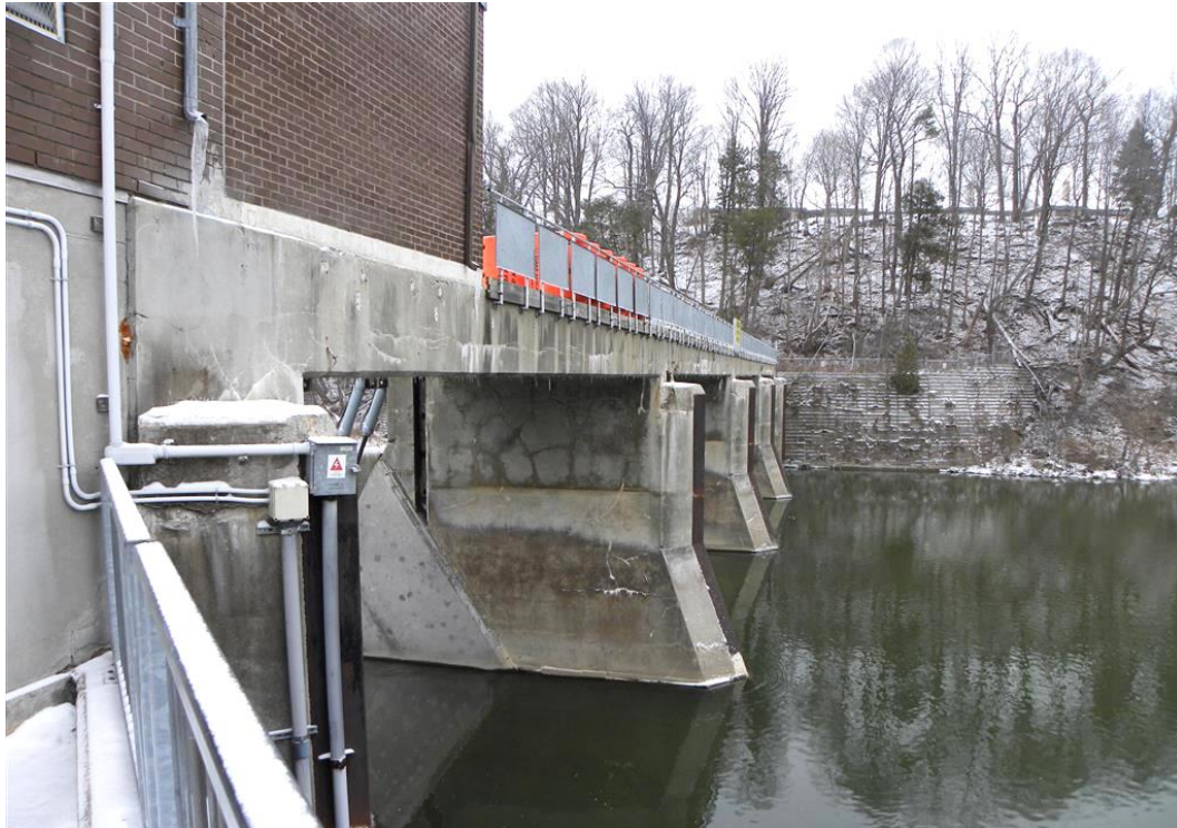
Figure 14: Detail of the east side of the Springbank Dam. Cement panels on the west side of the pier cover a groove where stop logs once rested (January 18, 2019).
