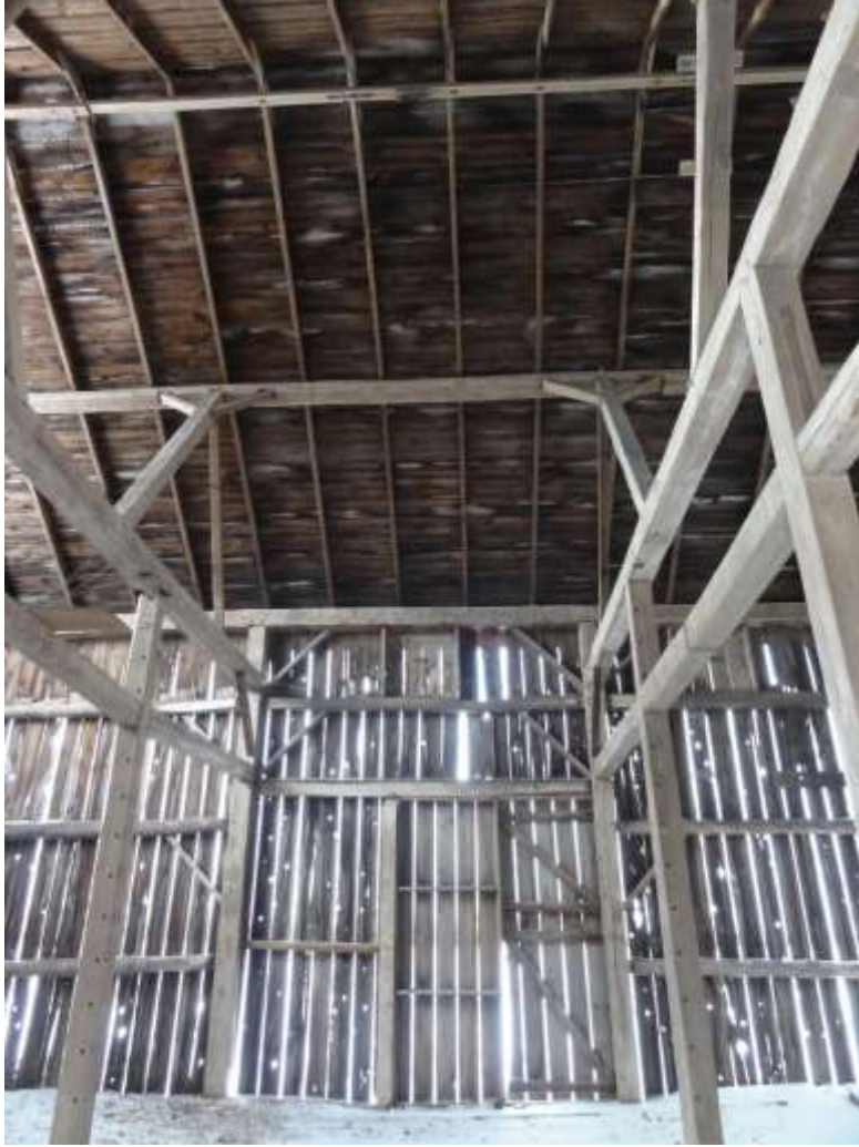
Image 5: View of barn interior illustrating structure, middle bay and timber framed bents (2019-02-14).
