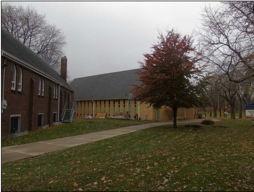
Image 11: St Andrew Memorial Church property with 1941 church at left, south elevation of 1957 at right. (AECOM, 2018)
