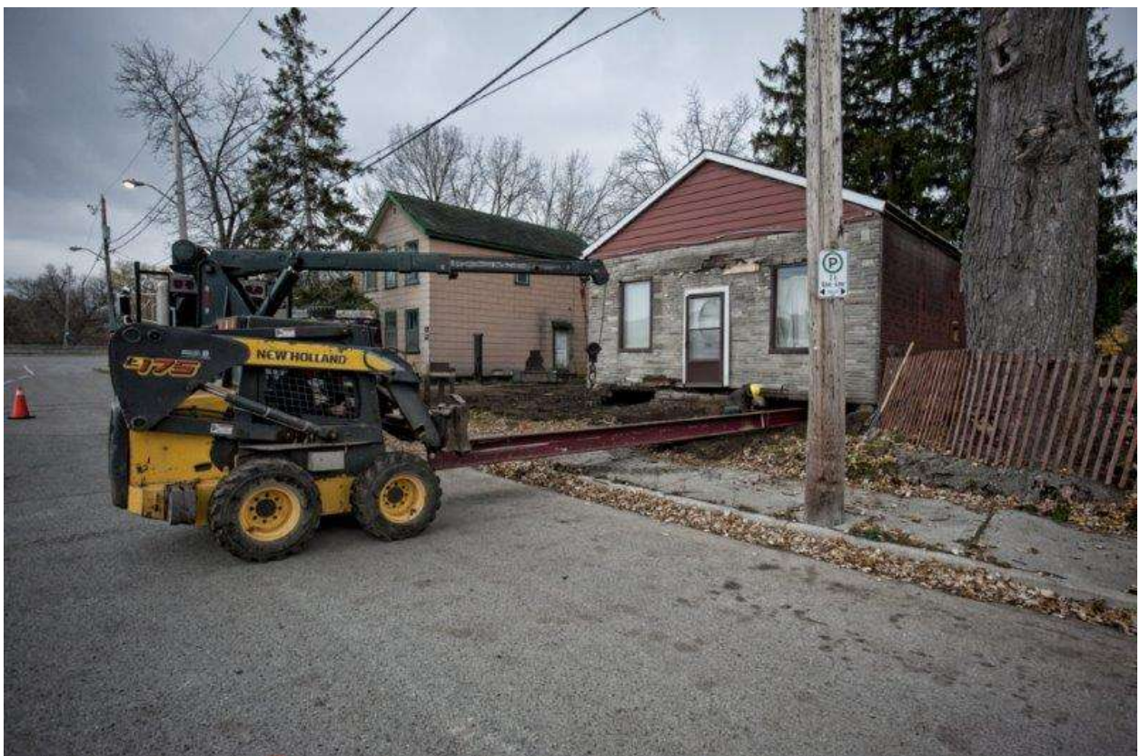
Image 4: Photograph of the building at 275 Thames Street on November 17, 2014 being lifted for relocation to 432 Grey Street
