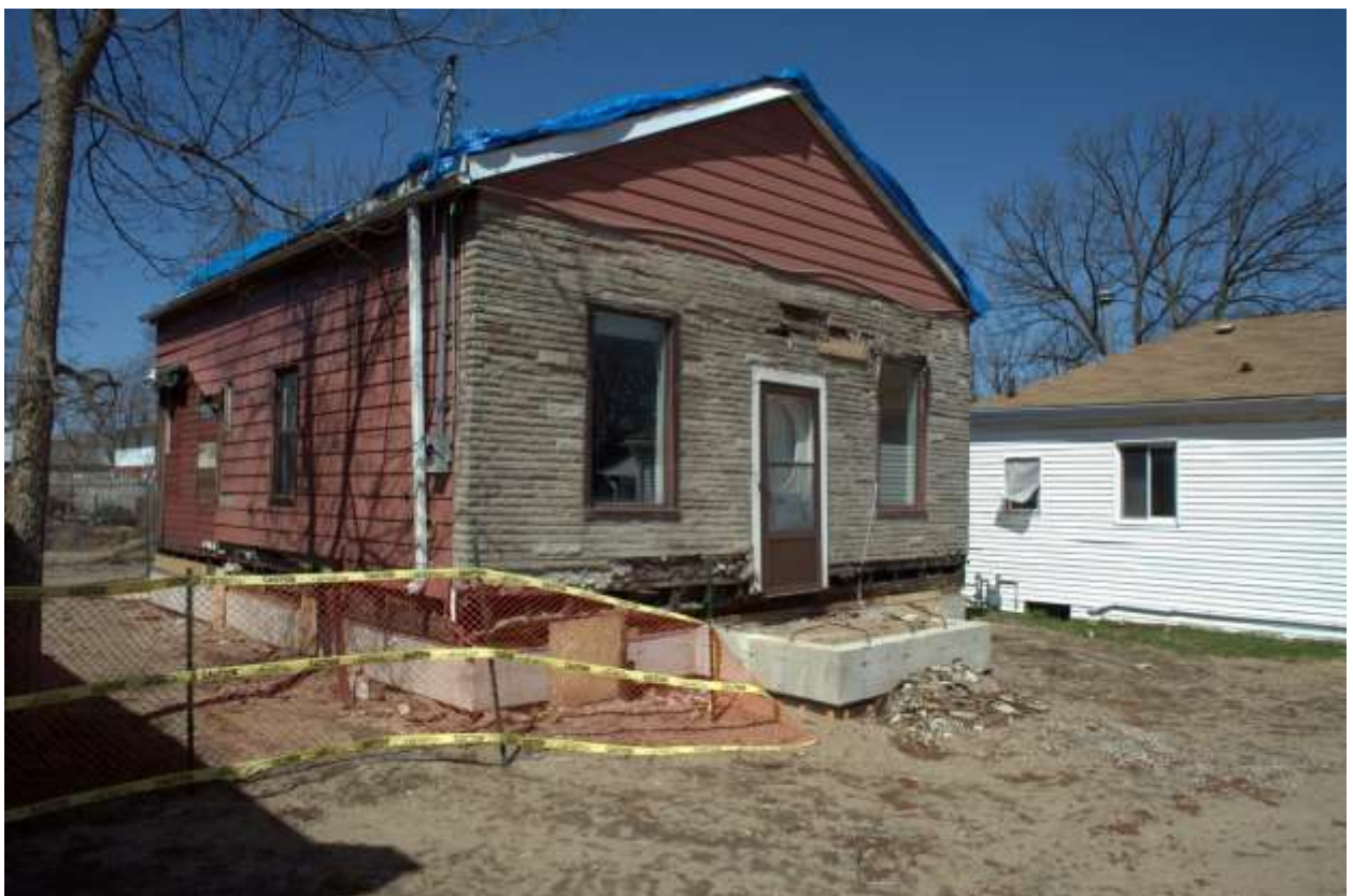
Image 6: Photograph of the Fugitive Slave Chapel building being position onto new concrete foundation at 432 Grey Street, April 24, 2015
