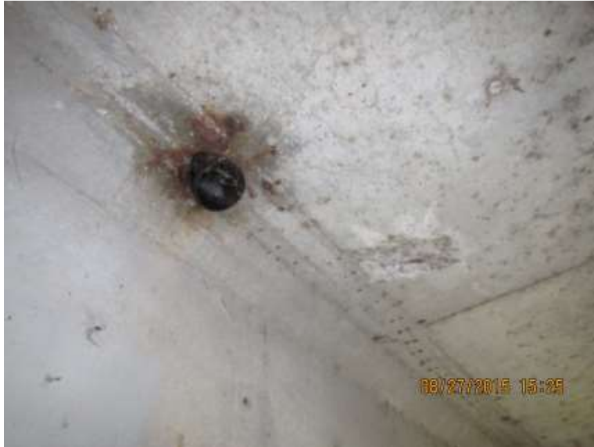
DECK DRAIN - AUG'15
