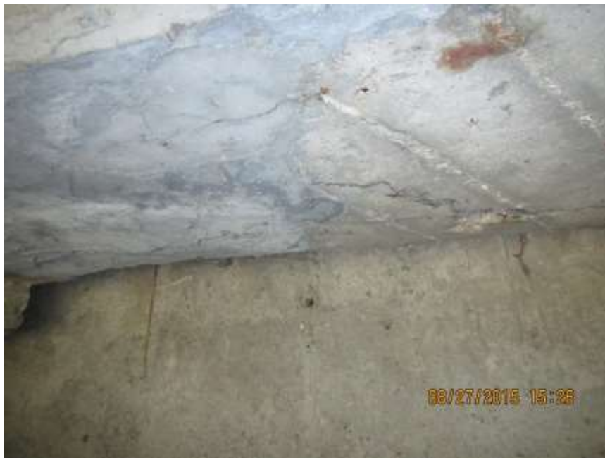
DELAMINATION AT DIAPHRAGM AT NORTH ABUTMENT - AUG'15
