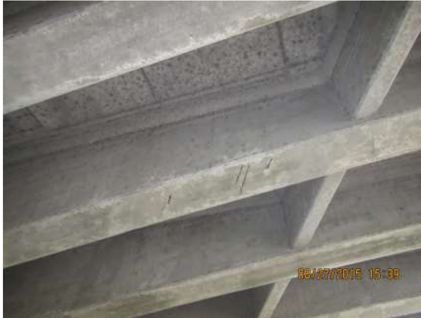
EXPOSED BARS ON GIRDERS - AUG'15
