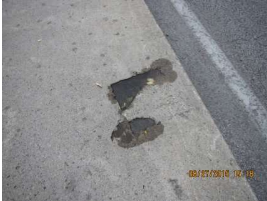
SPALL IN WALKWAY - AUG'15
