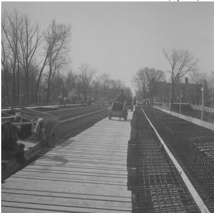
Figure 17: Pouring cement at Wharncliffe Road Bridge, view south Source: LFP Collection of Photographic Negatives, Western Archives, April 14, 1958
