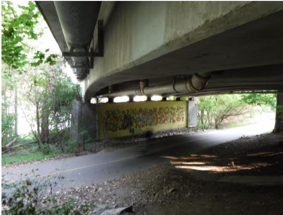
Plate 17: View of the south face of the south pier from the abutment.
