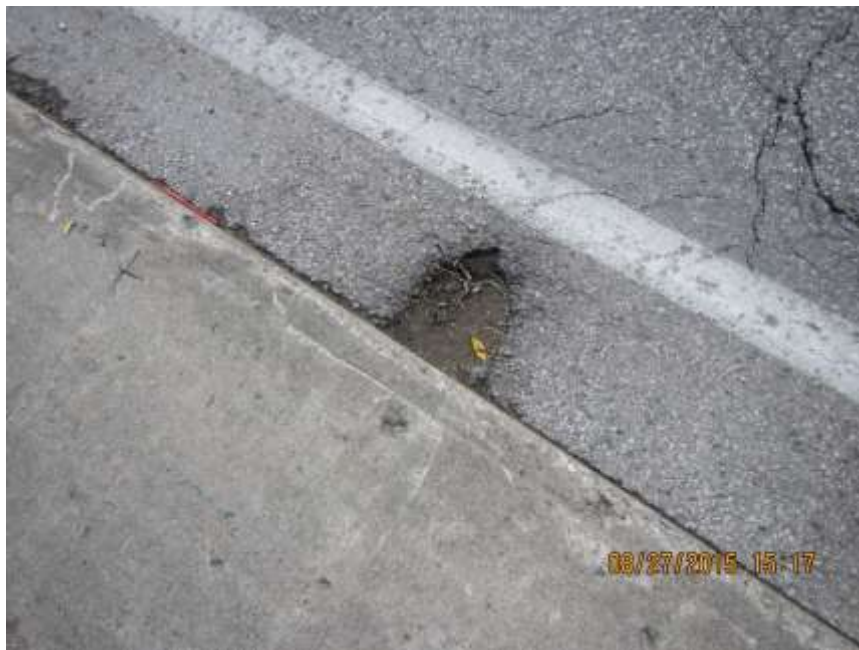
BLOCKED DECK DRAIN - AUG'15
