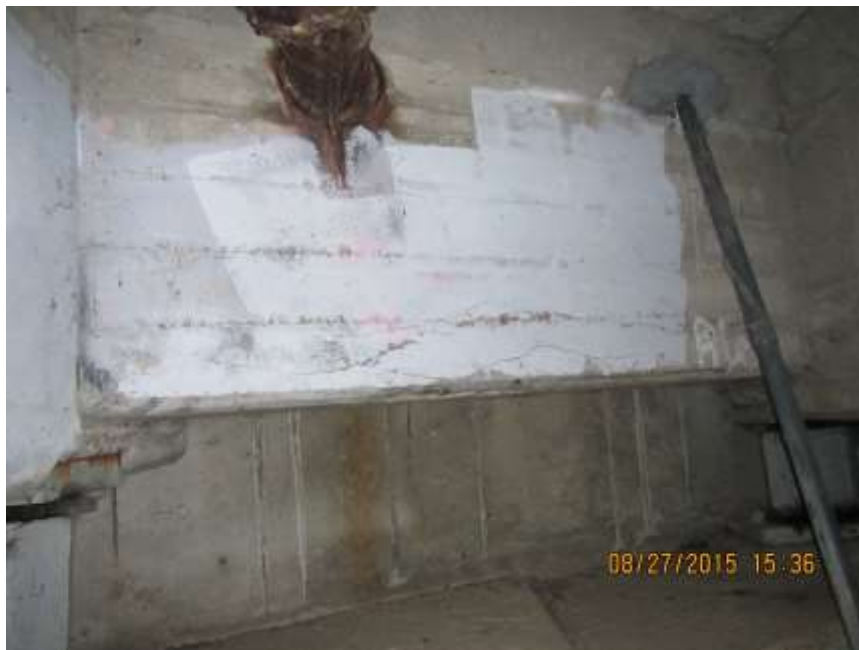
CRACKING AT SOUTH DIAPHRAGM - AUG'15
