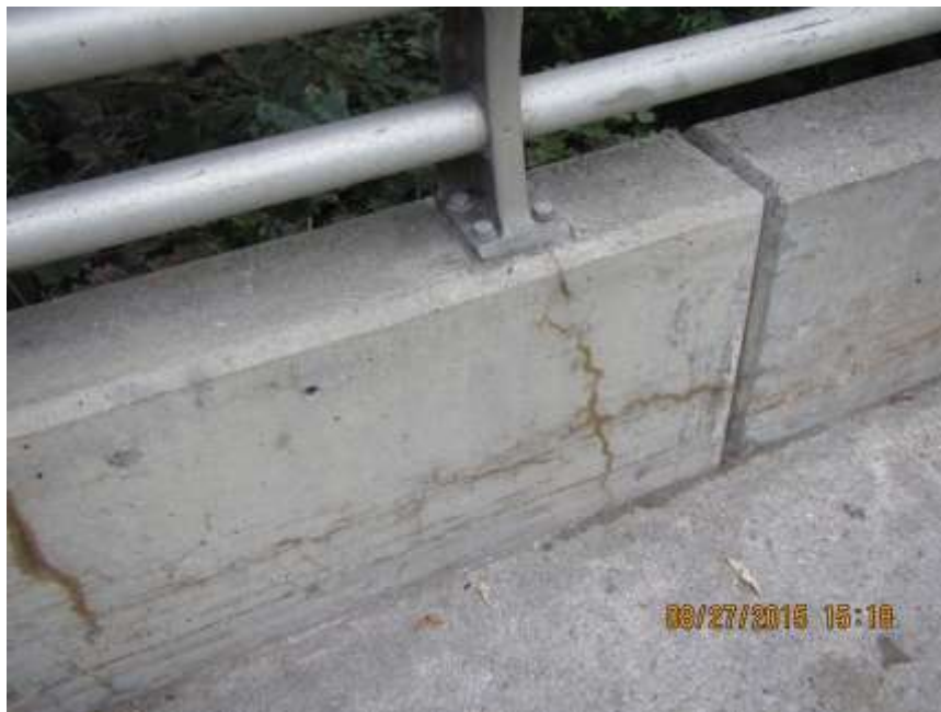
CRACKING AT PARPET WALL - AUG'15
