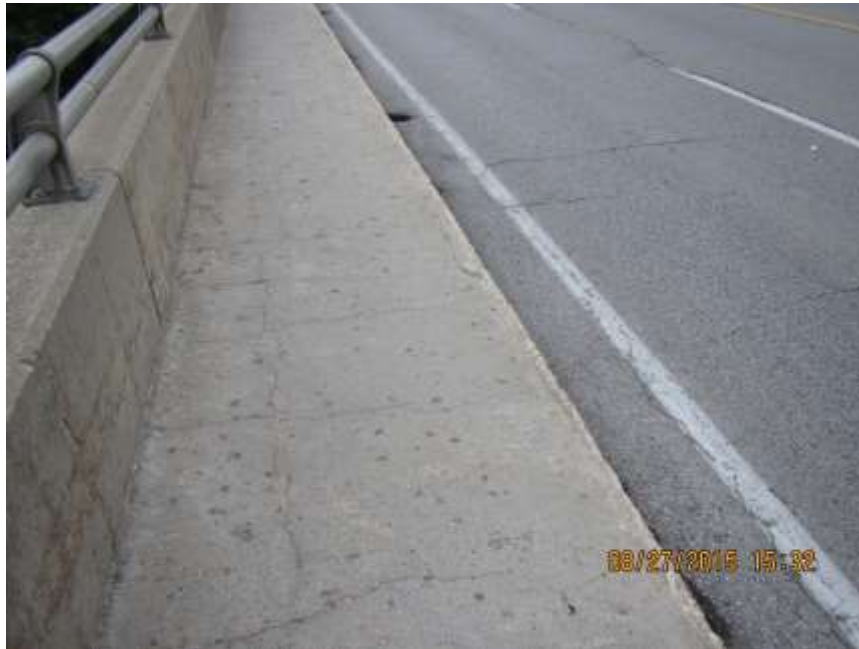
CRACKING AT SIDEWALK - AUG'15
