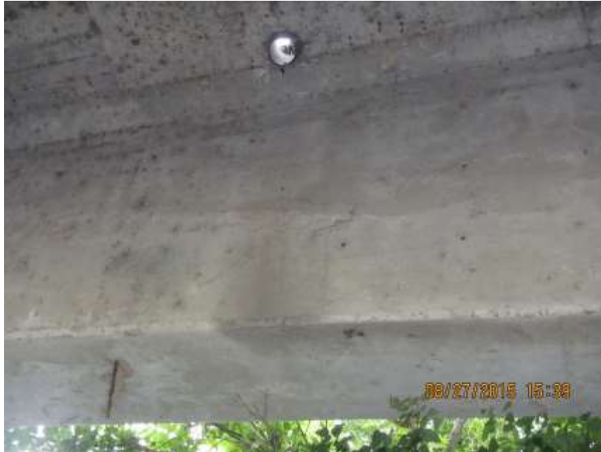
DELAMINATION ON GIRDER - AUG'15
