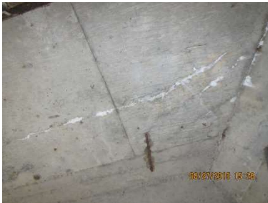
STAINED CRACKS IN SOFFIT - AUG'15
