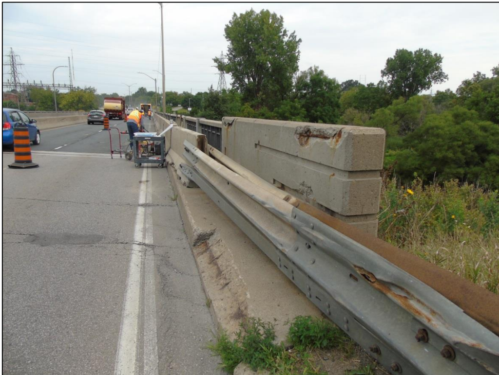
Photograph 21: View showing deck with asphalt wearing surface, concrete curbs, as well as temporary concrete barriers
