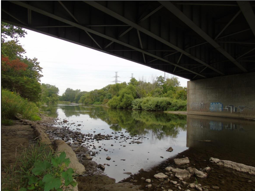
Photograph 3: View looking upstream from under the bridge showing centre pier at right and north banks at left
