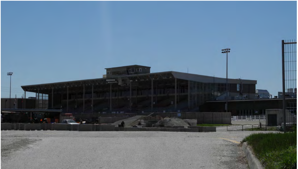
Figure 49 - Looking southwest onto the open seating area of the Grandstand structure from inside the Racetrack (CBCollective 2018).
