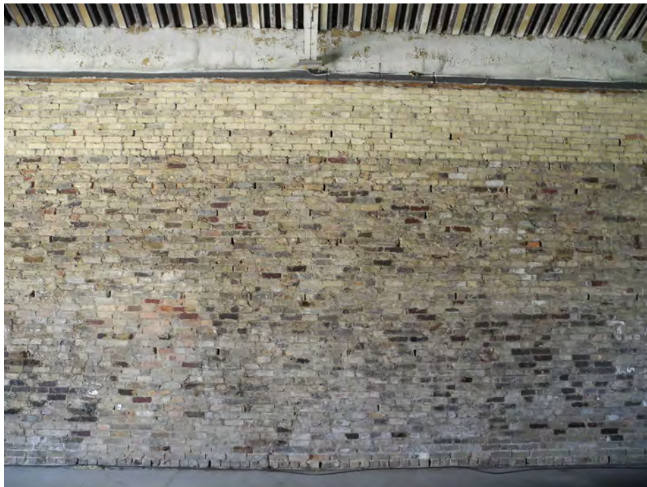
Figure 30 - Interior wall of the Arts Building, presently unfinished. The different types of bricks used are apparent, and the steel roof and truss system is visible at the top (CBCollective 2018).
