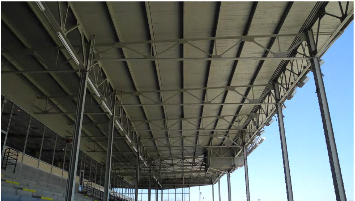
Figure 50 - The Grandstand support structure dates from 1915, and uses steel piers supporting trusses comprised of riveted girders (CBCollective 2018).
