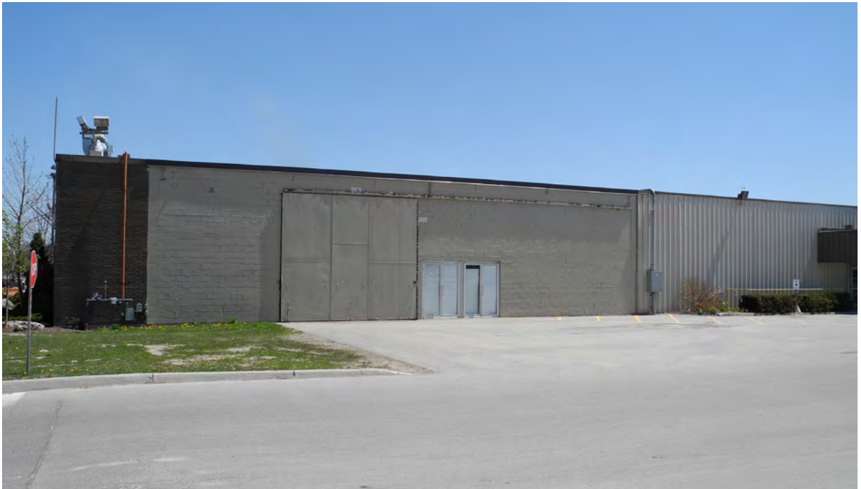
Figure 47 - Scarring and sliding door on the west wall of the Canada Building indicate where the Link connected it with the Poultry Building until 2013 (CBCollective 2018).
