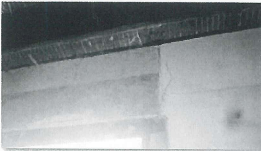
Image 30: Cracking at Window
