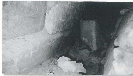
Image 4: Penetration in Exterior Brick Wall at base.
