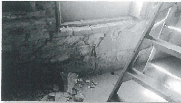
Image 26: Cracked Brick wall at Window
