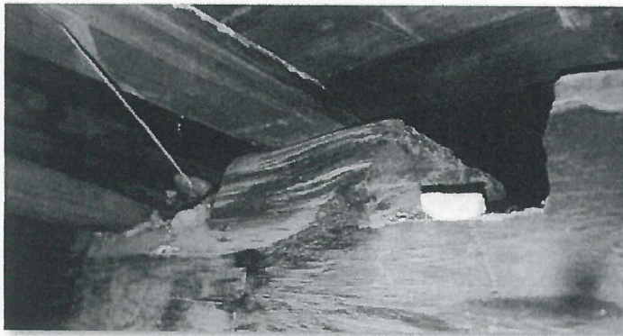
Image 20: Cut joist at rear of house.
