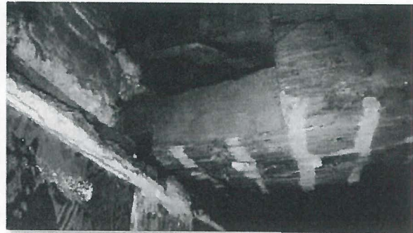
Image 27: Cut floor joists and minimal bearing at brick wall
