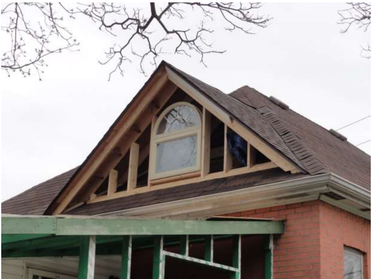
Image 2: Close-up view of partially constructed rear dormer (west) at 104 Wharncliffe Road North (May 11, 2018)
