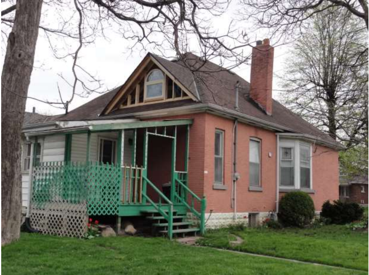
Image 1: View of partially constructed rear dormer (west) at 104 Wharncliffe Road North (May 11, 2018)
