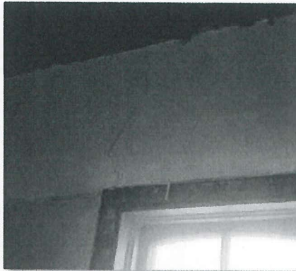
Image 29: Cracking at Window
