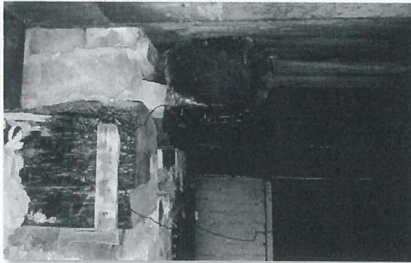
Image 10: Basement Beam near stair cut. Floor joist has no support
