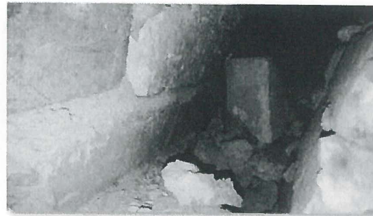
Image 4: Penetration in Exterior Brick Wall at base.
