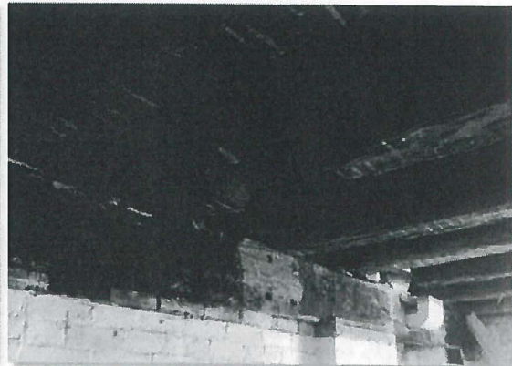
Image 13: Joist below main entrance cut. Floor joist has no support
