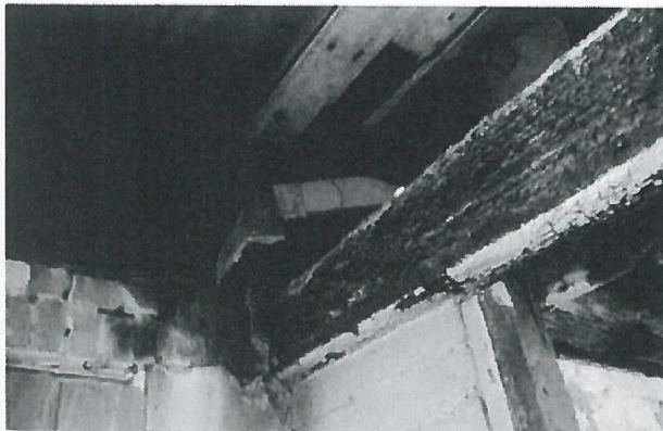
Image 12: Joist near stair cut. Floor joist has no support
