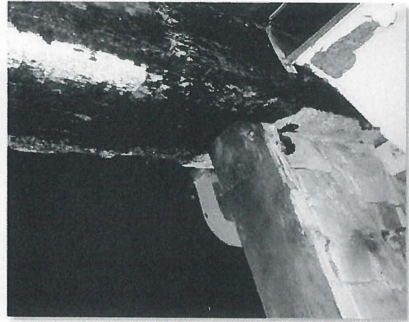
Image 11: Charred beam eccentrically placed On single Wythe brick below.
