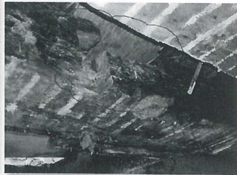
Image 21: Charred and cut joist at rear of house.
