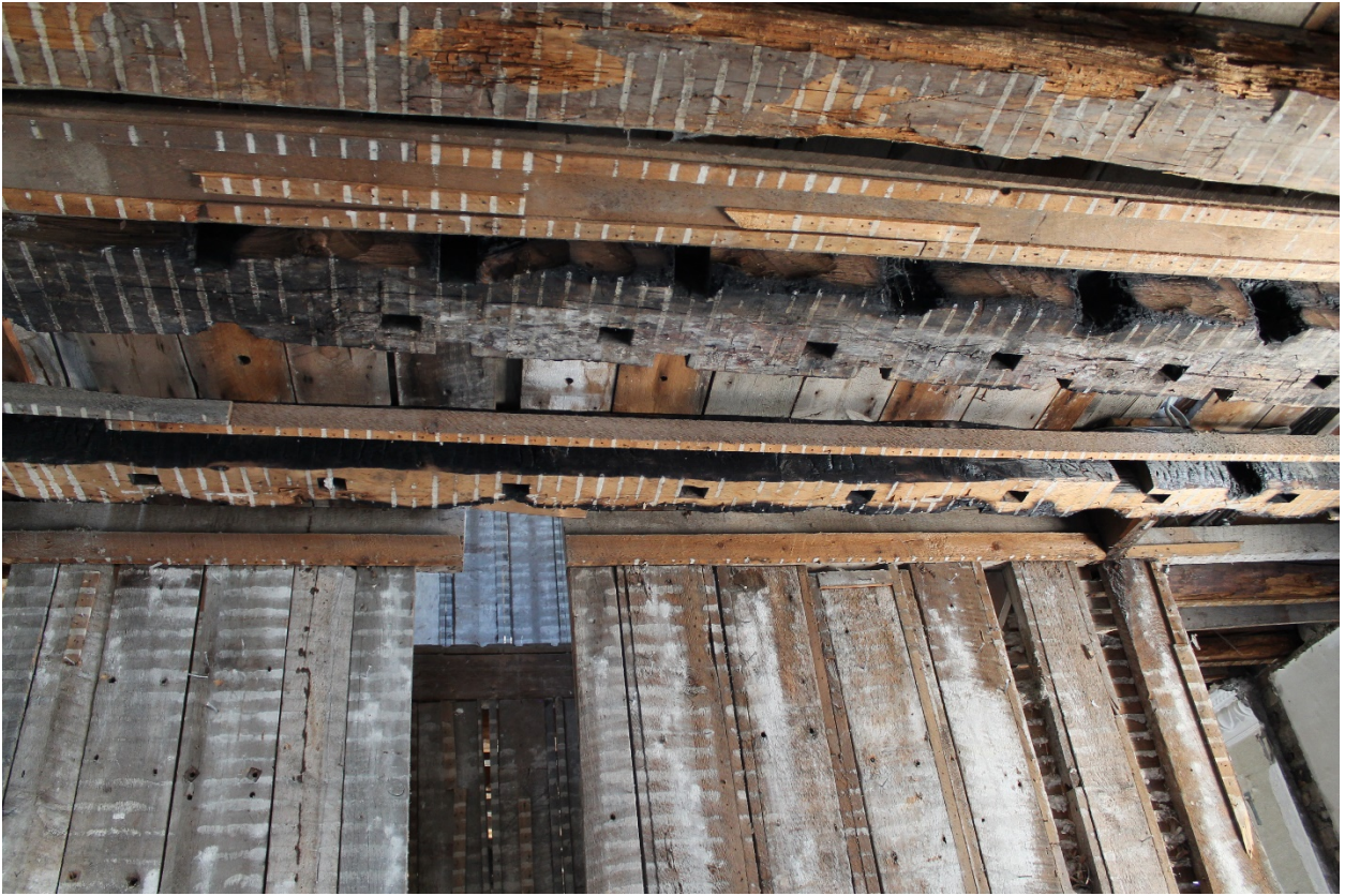
Image 7: Photograph of the interior of the building at 172 Central Avenue; lath and plaster has been removed to reveal the structure of the building. Note the inconsistent charring of the timber members, which suggests that the wood was charred before its assemblage in this building (May 1, 2018).
