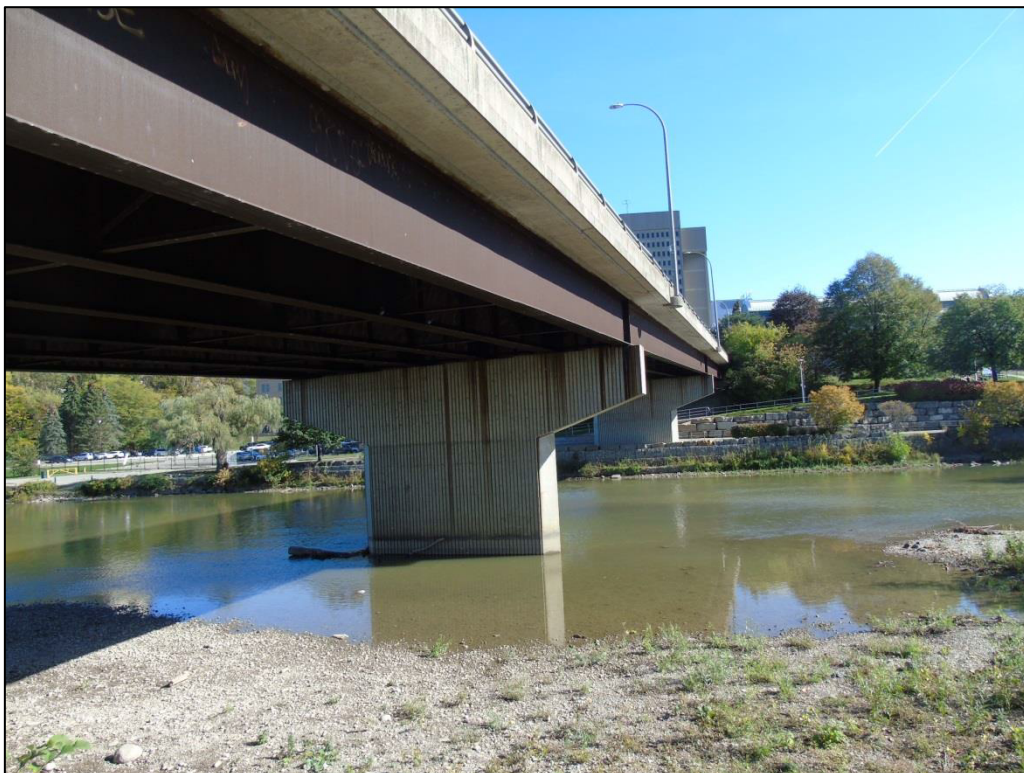
Image 19: View looking east across the river, showing piers supporting the steel girders
