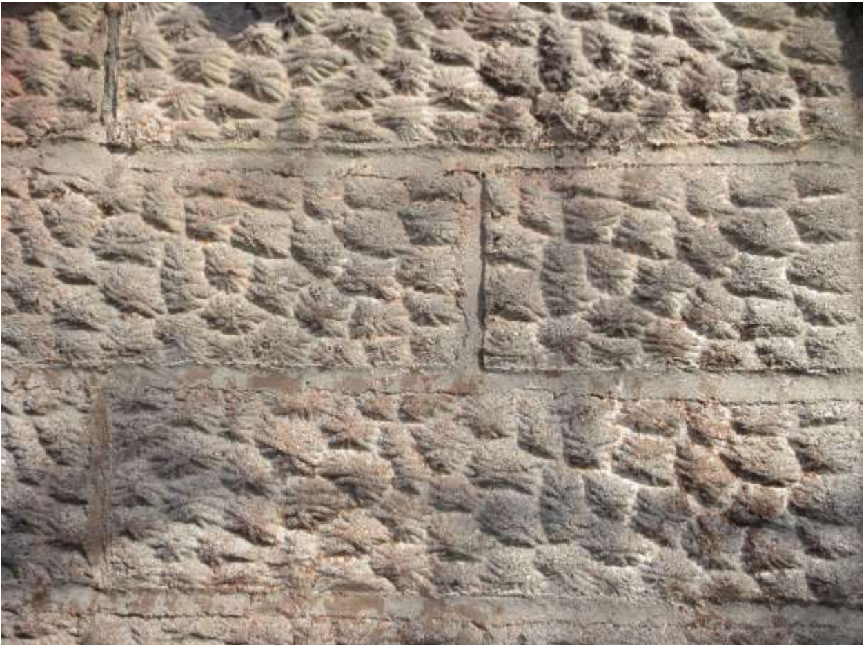
Image 14: Detail of the cast concrete block which comprises the base of the barns located at 2154 Richmond Street.
