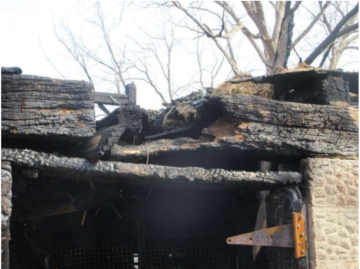
Image 15: Detail of the damage caused by fire on February 16, 2018 to the south barn located at 2154 Richmond Street.
