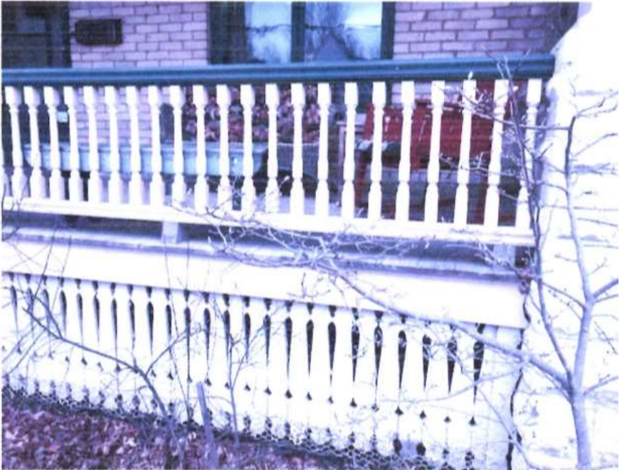
Image 7: Detail of balustrade of porch of the building at 846 Princess Avenue; height of balustrade ties into capstone of the cast concrete piers
