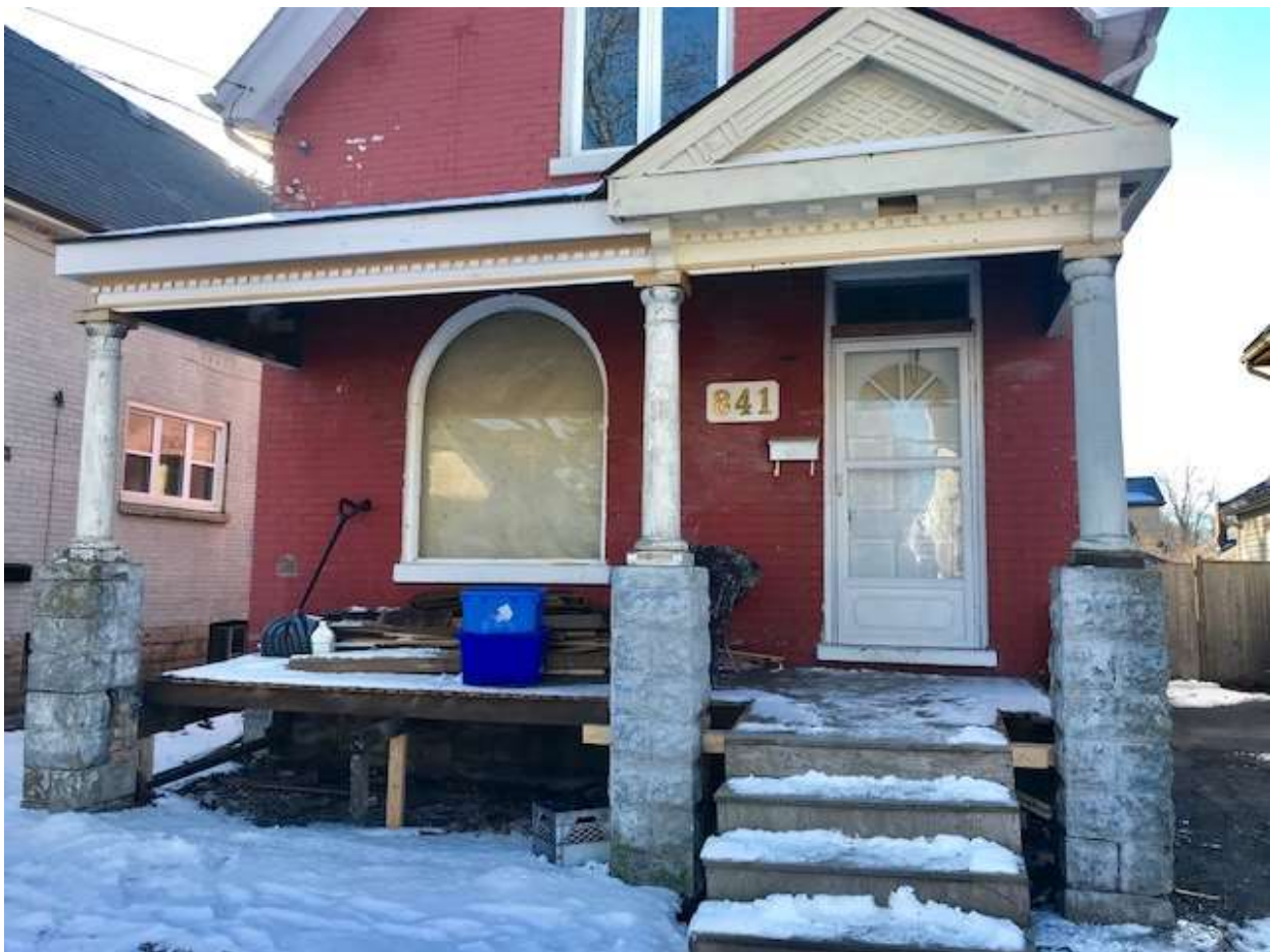
Image 2: View of the property located at 841 Princess Avenue after removal of portions of the existing porch (March 5, 2018; by applicant)
