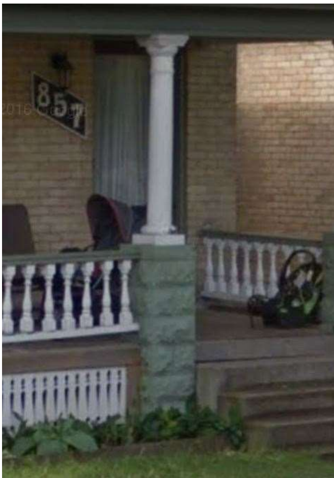
Image 6: Detail of balustrade of porch of the building at 857 Princess Avenue; height of balustrade ties into capstone of the cast concrete piers
