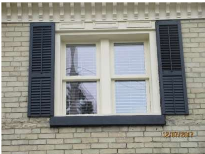
Image 9: Detail of the front window in the upper storey of the building located at 33 Beaconsfield Avenue (December 7, 2017). Note the absence of wood trim detail on the mullion.
