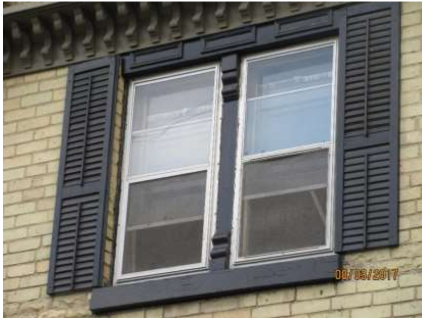
Figure 4: Detail of original mullion detailing of the upper windows of the building located at 33 Beaconsfield Avenue, which will be used to replicate the lost detailing in wood.
