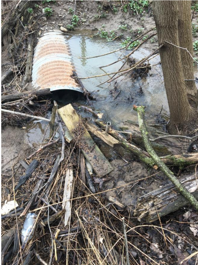
Figure 1. Image of the partially buried culvert on the north side of Southdale Road. The image shows a large build-up of detritus causing the burying of the opening and restricting fish passage.
