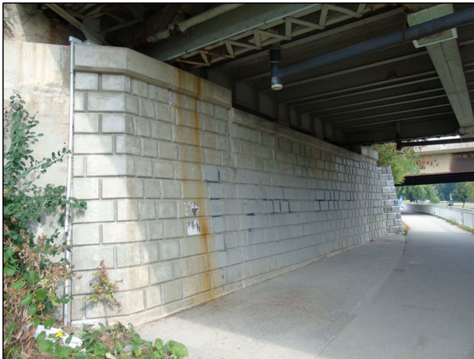
Image 26: West abutment showing concrete block designed to appear as stone pattern, consistent with dyke walls
