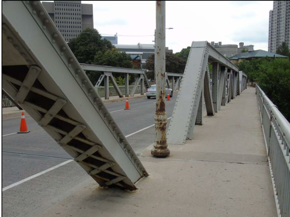
Image 38: View showing base of lighting systems in the centre of the bridge
