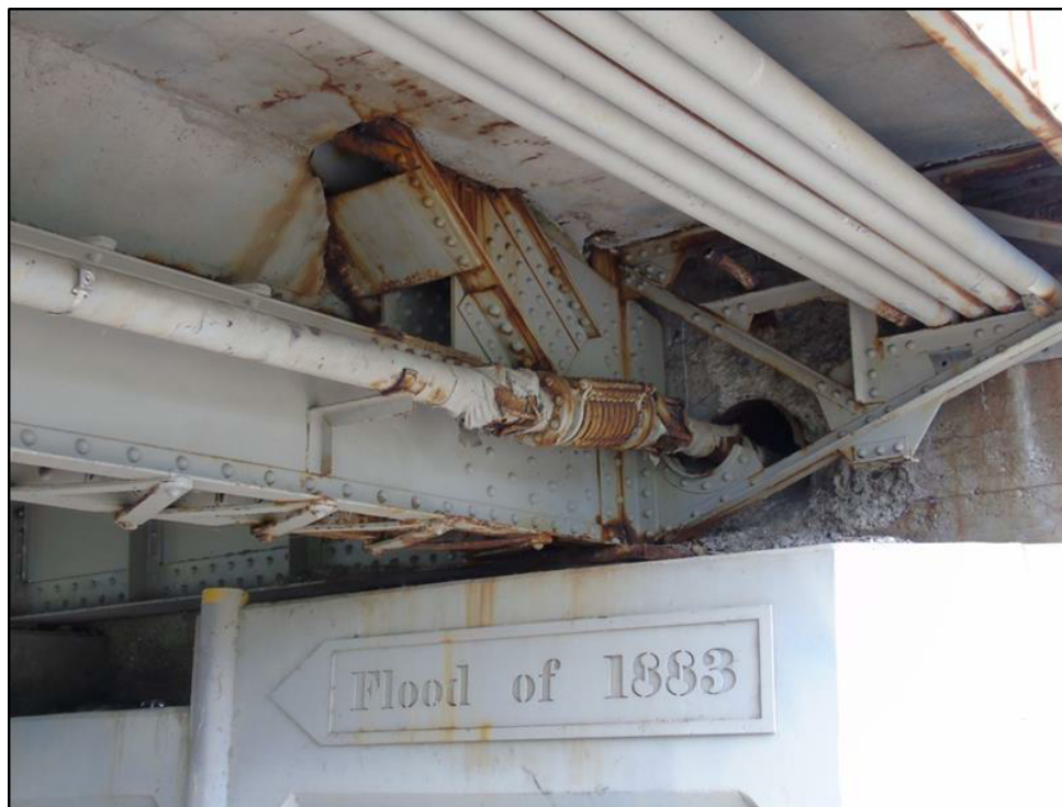
Image 23: Detail of "Flood of 1883" markers on east abutment, as well as connection of bottom chord
