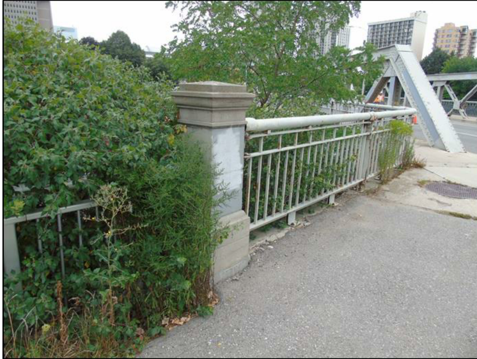
Image 36: Railings and concrete end post at west end of the bridge. The end post appears to be a small version of the large concrete end posts that were once located at each end of the bridge
