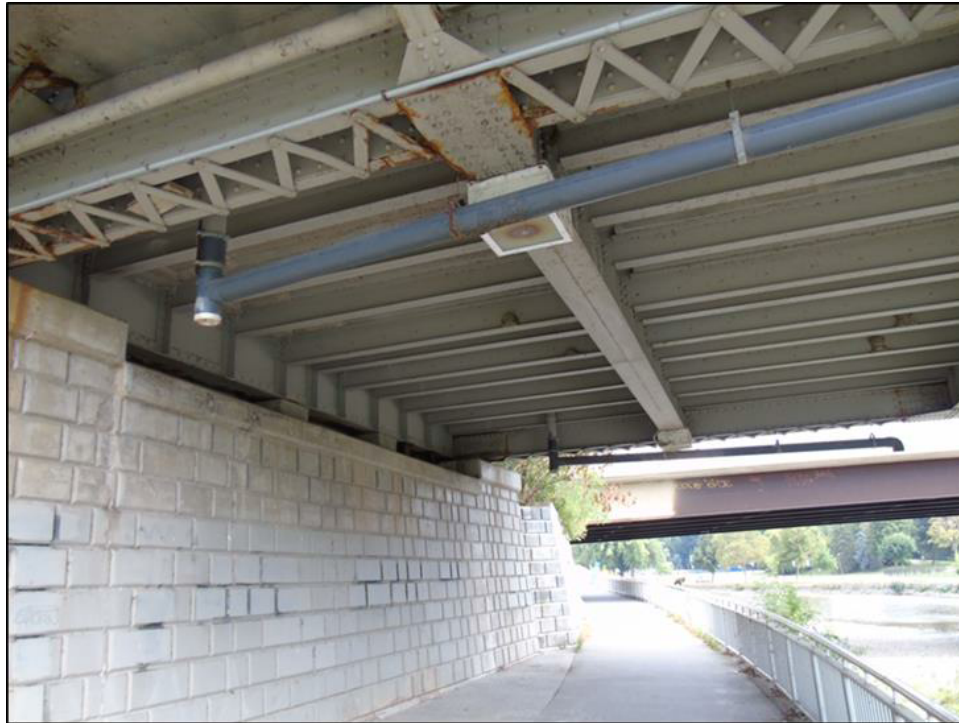
Image 16: View looking north from west abutment showing TVP built into the West London Dyke system on the west side of the river
