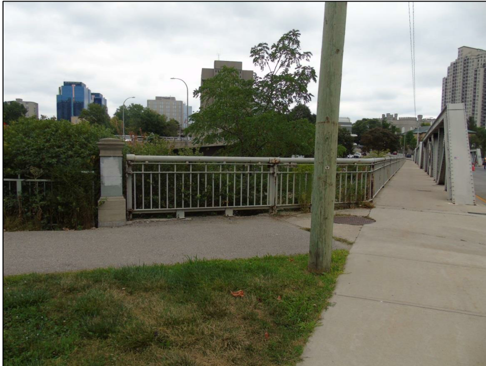
Image 37: View showing concrete end post for railing system at west end of the bridge
