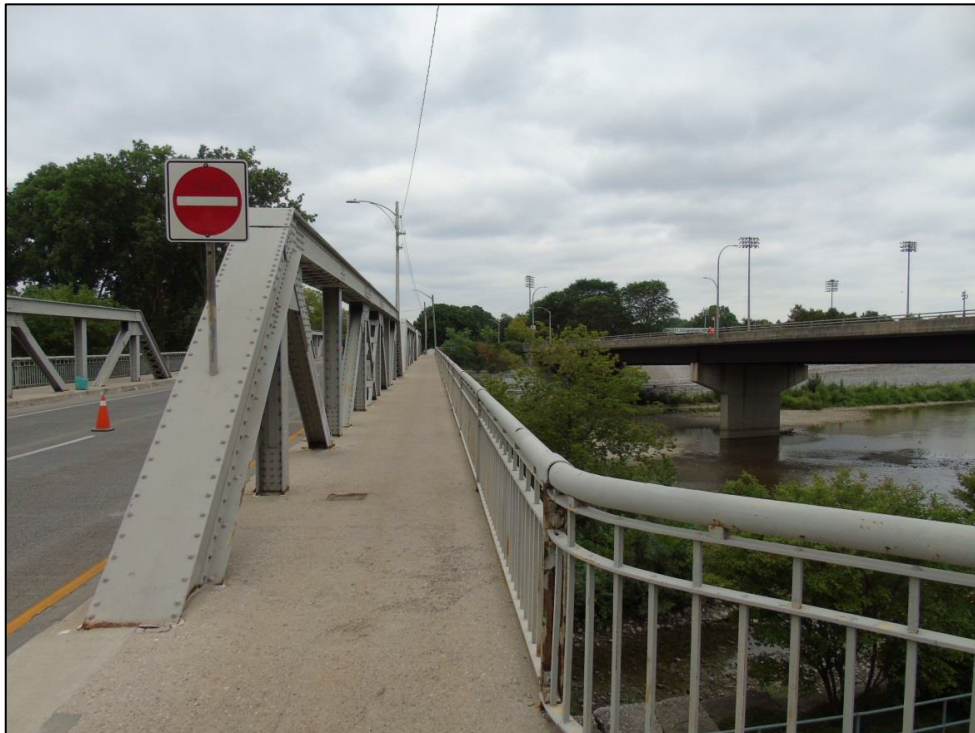
Image 36: View looking west across the bridge showing deck, concrete sidewalks, and railing system
