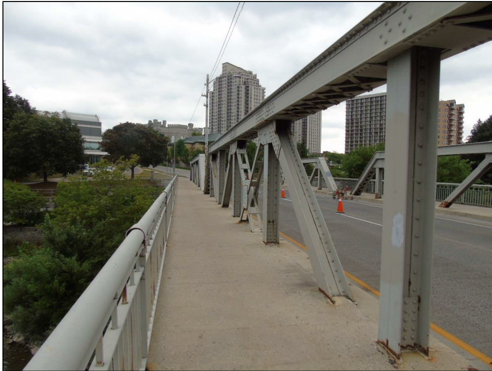
Image 28: View looking east showing top chord, verticals, and diagonal members of the truss system
