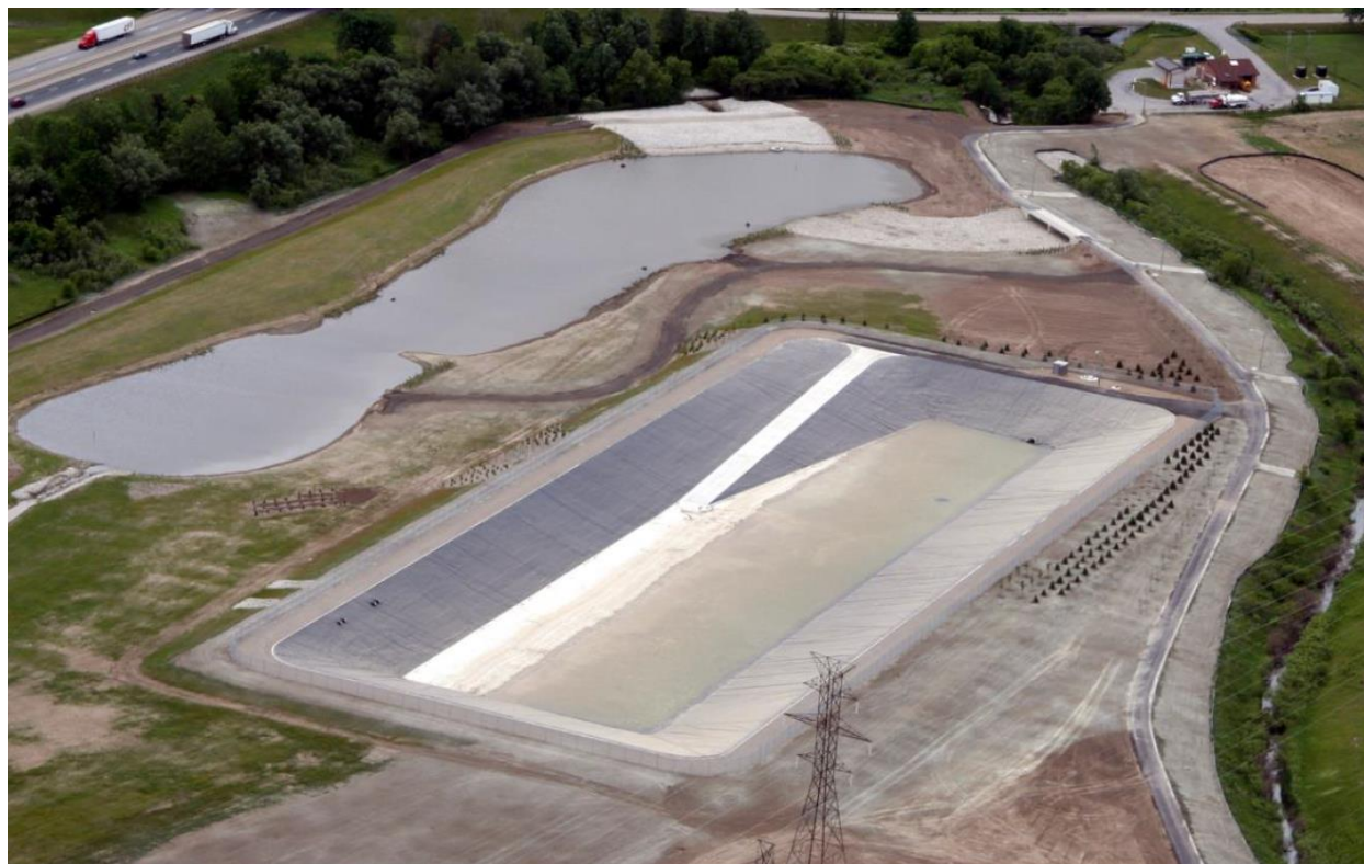
Figure 2 – Dingman Creek Storage Facility
