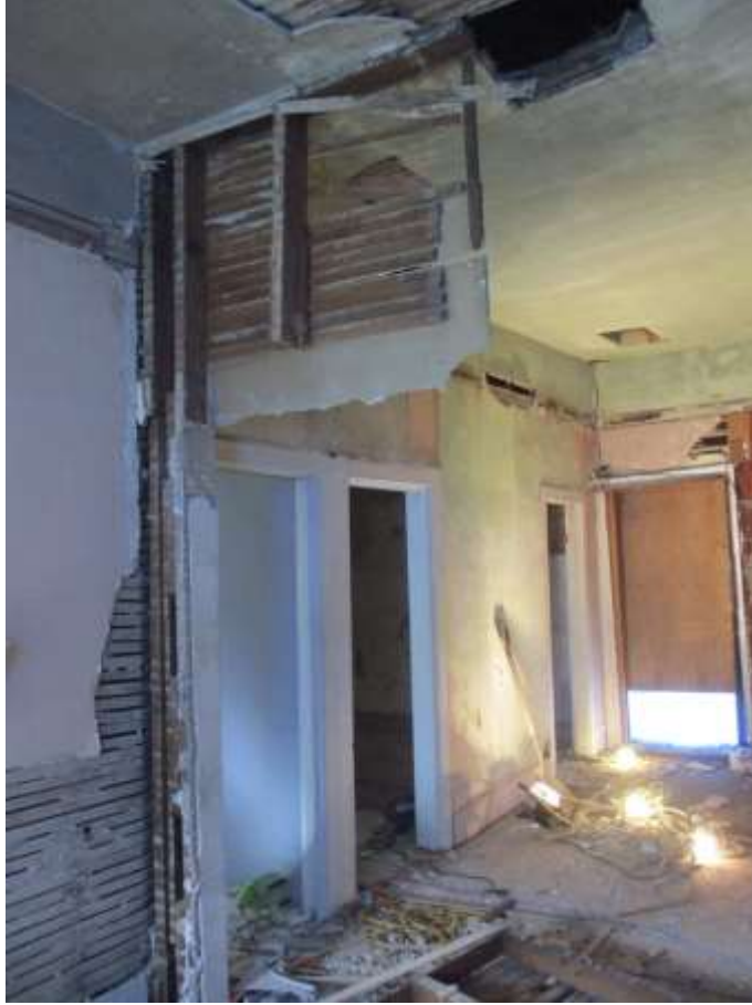
Looking along the north-south wall as it extends towards the rear of the building
